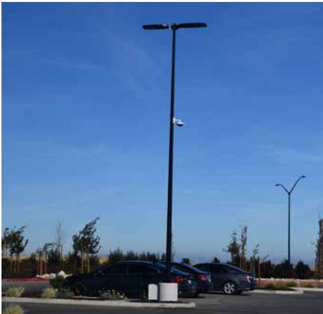
Typical Double-Head Parking Lot Lighting
