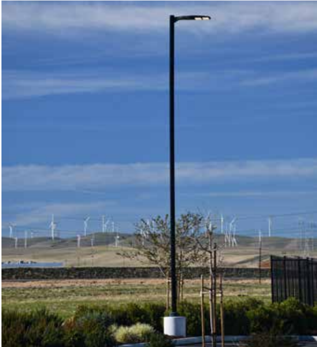
Typical Single-Head Parking Lot Lighting
