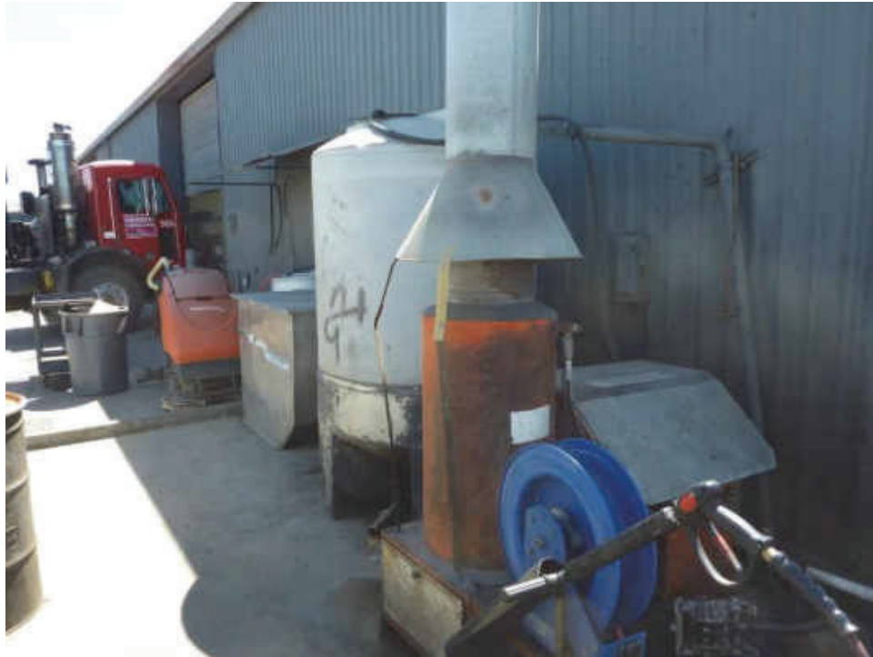
E-27. Steam cleaning equipment and aboveground clarification system behind (southwest of) maintenance building at 1535 Industrial Avenue (06/22/2020).
