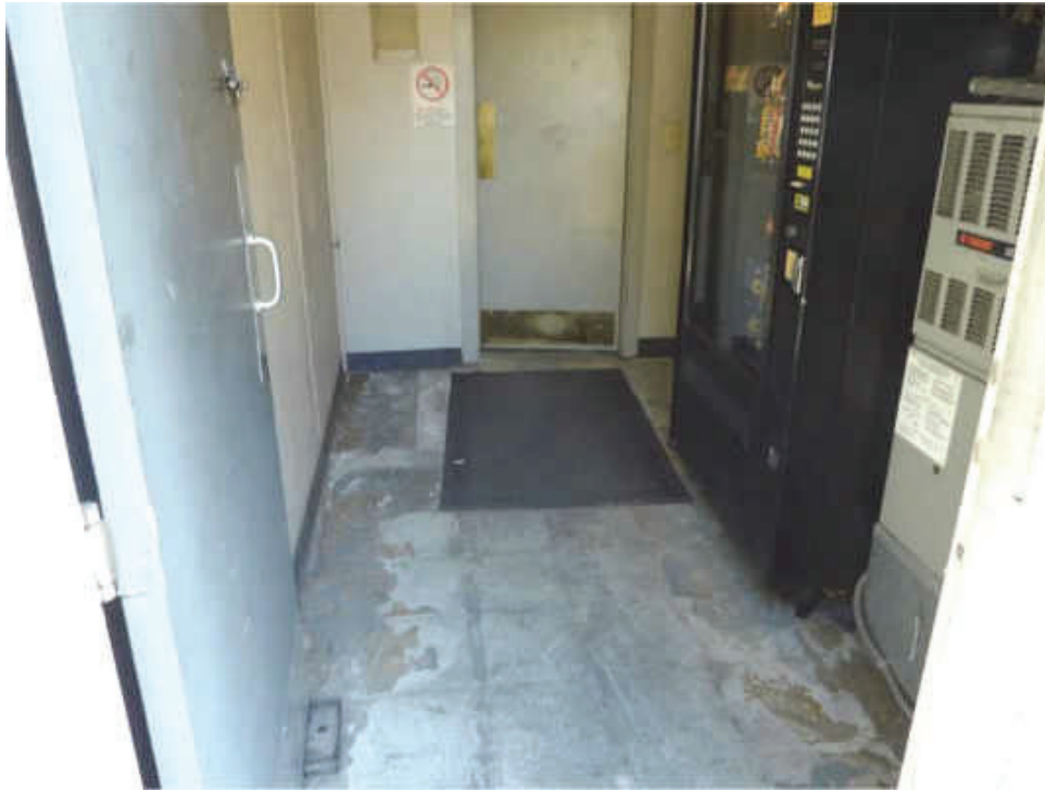
E-3. Looking northeast into vending machine area and restrooms at FJM office building at 1535 Industrial Avenue with evidence of former 12-inch VFT (06/22/2020).
