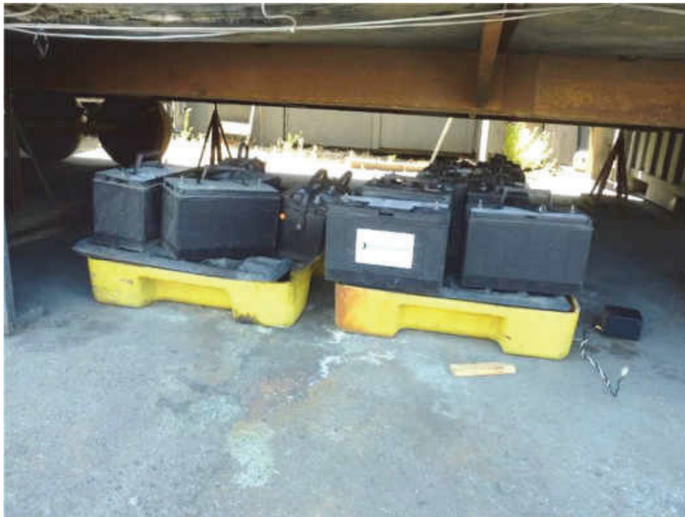
E-30. Battery storage beneath rear of FJM modular office structure at 1575 Industrial Avenue (06/22/2020).
