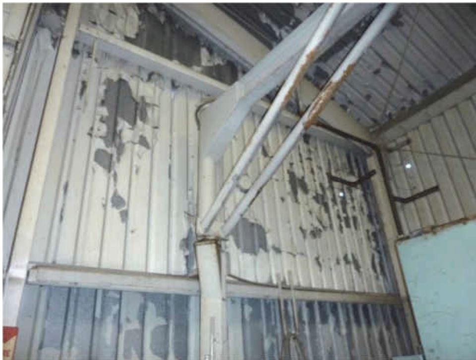
E-16. Damaged and peeling paint on inside of gable wall and underside of roof in maintenance shop at 1535 Industrial Avenue (06/22/2020).
