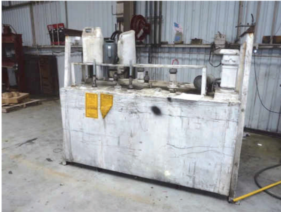
E-35. AST for waste oil inside truck repair shop at 1535 Industrial Avenue (06/22/2020).
