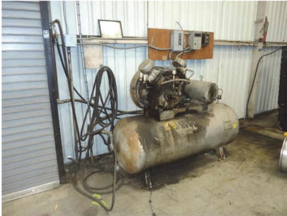
E-33. Air compressor inside southwest wall of truck repair shop at 1535 Industrial Avenue with oily residue on floor beneath (06/22/2020).
