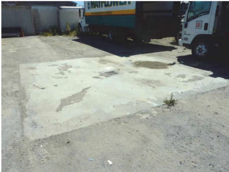
E-38. Looking northeast at suspected steam clean slab behind maintenance shop at 1575 Industrial Avenue (06/22/2020).
