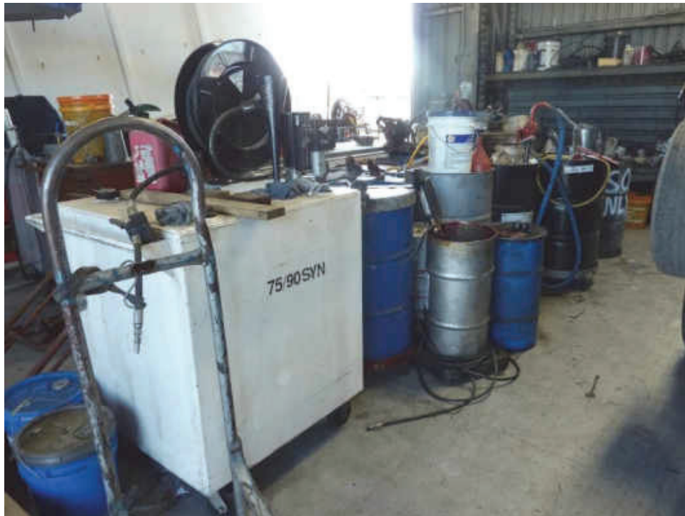
E-9. Looking southeast at mobile AST for synthetic oil with drums of oil and grease in background in maintenance shop at 1535 Industrial Avenue (06/22/2020).
