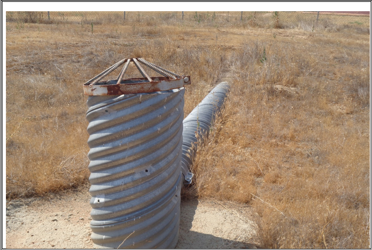
Photograph Number 13: drainpipe associated with the catch basin.
