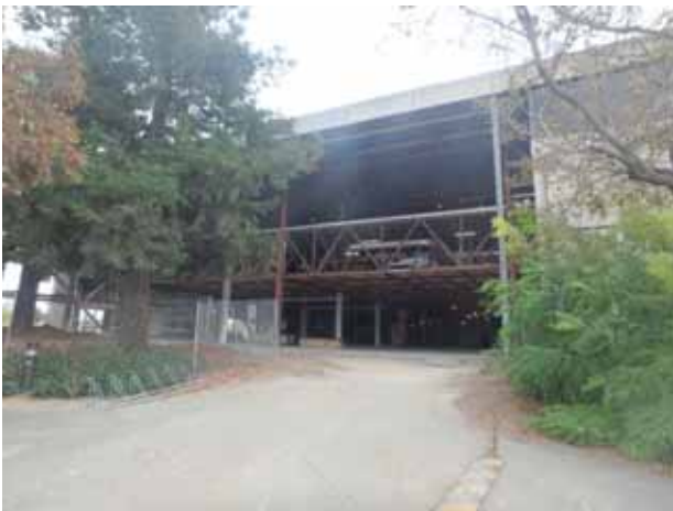
15. View of the southeastern portion of the Lumileds building to the southwest of the subject property, currently being renovated
