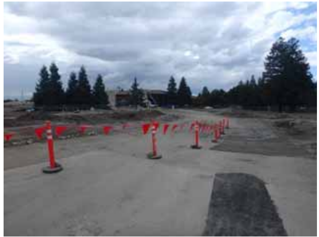
10. View of the construction entrance to the subject property from Orchard Parkway to the east
