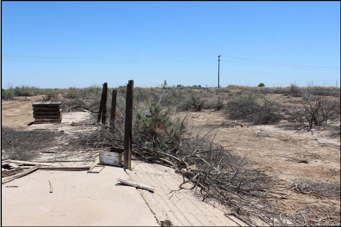
Photo 9: Close-up view of concrete lined basin in the northeast corner of the subject site.
