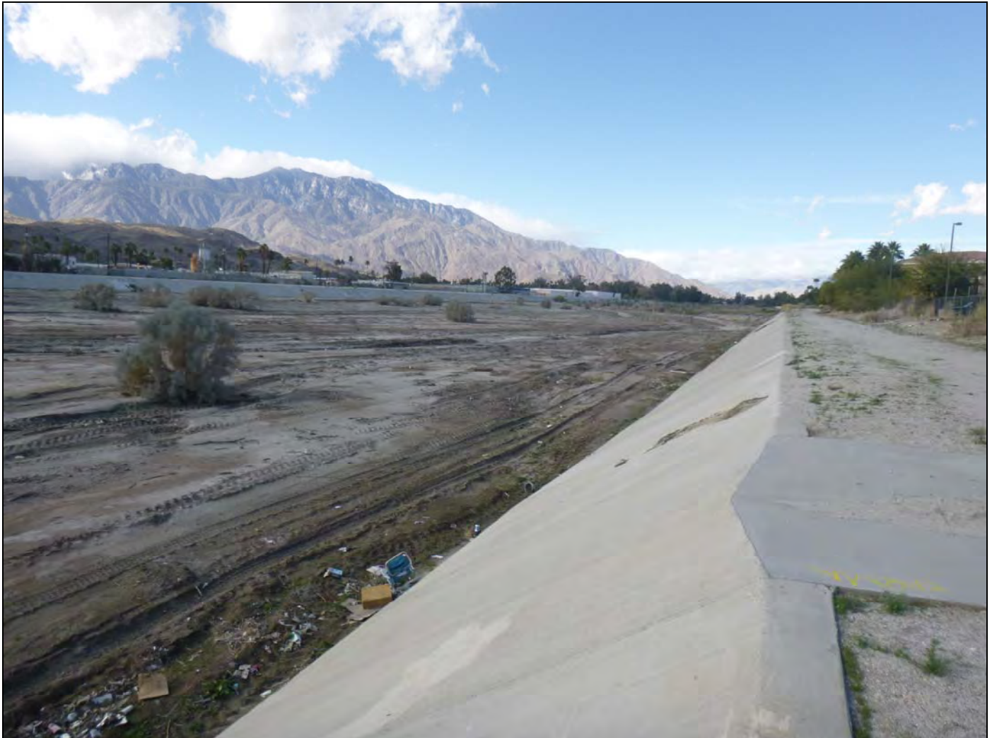
Channelized segment of the CVSC with cement-lined slopes between Frank Sinatra Drive and Cathedral Canyon Drive (view to the northwest; photograph taken January 10, 2017).
