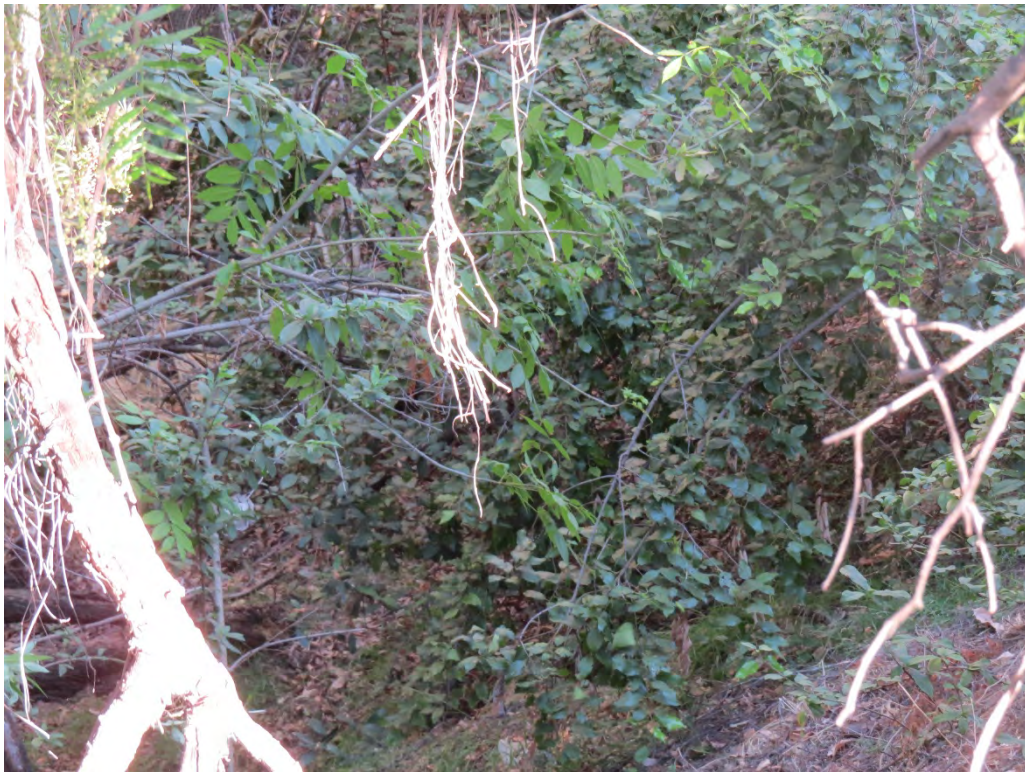
Photograph 10: Another view of the drainage feature on the south side of Palos Verdes Drive North.
