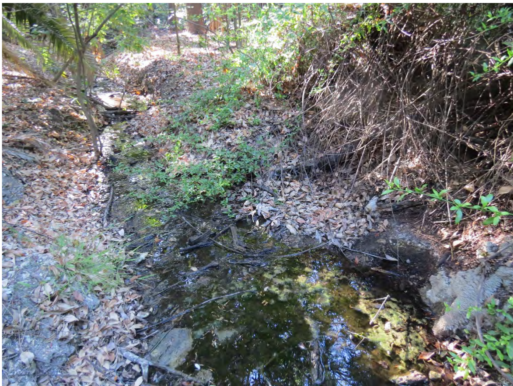
Photograph 12: Water ponding at the beginning of the drainage feature on the north side of Palos Verdes Drive North.
