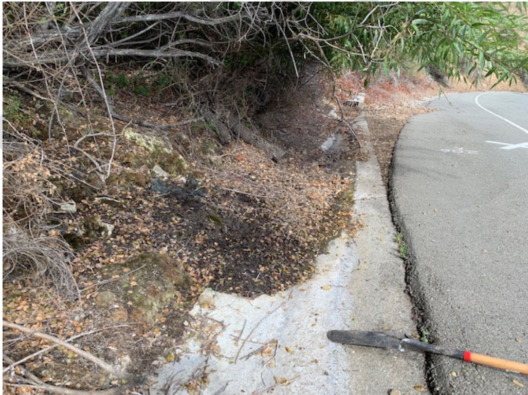
Appendix C-2. Concrete roadside ditch along Santos Ranch Road, below WS, with culvert inlet downstream in upper portion of photo, looking downstream (north).
