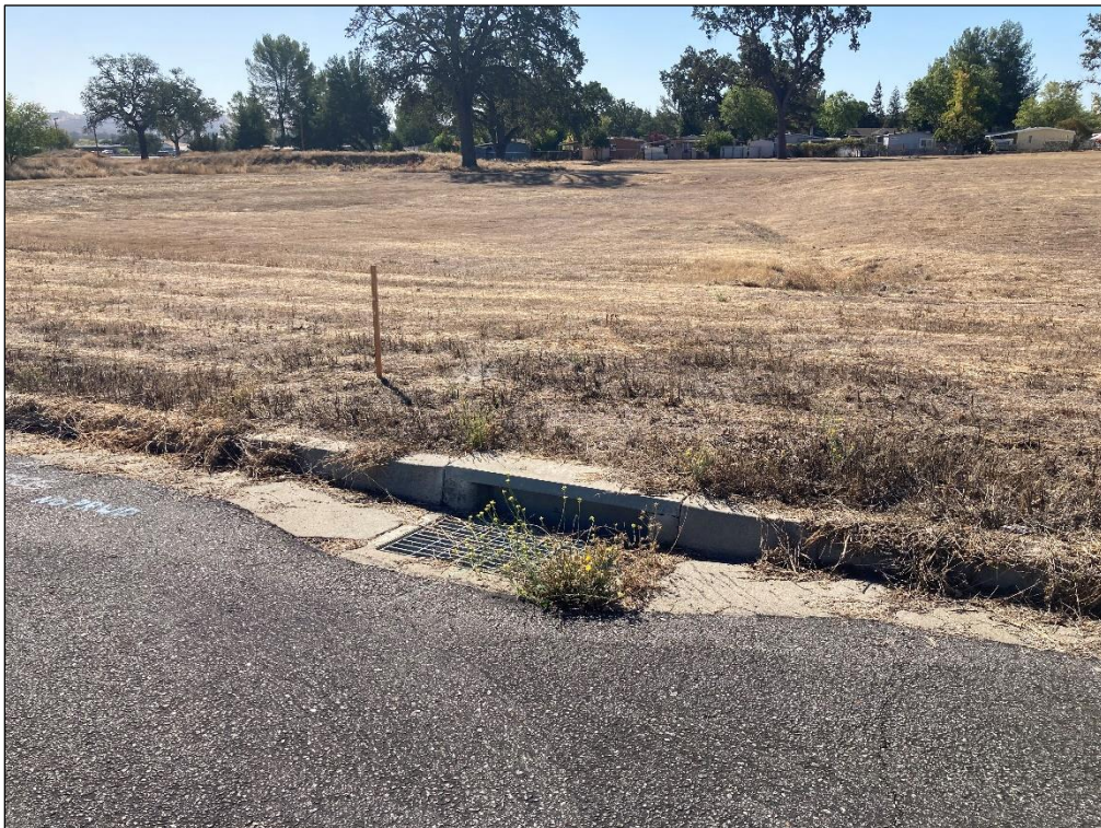
Photo 4. View from Nutwood Circle; drain leading to culvert pipe to direct flow into shallow man-made basin within the BSA (aspect southeast; 9/30/22).
