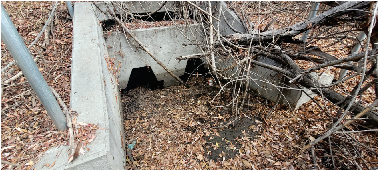
Photo 2: View looking at the box culvert located on the western end of Drainage 1. Photo Date September 15, 2022
