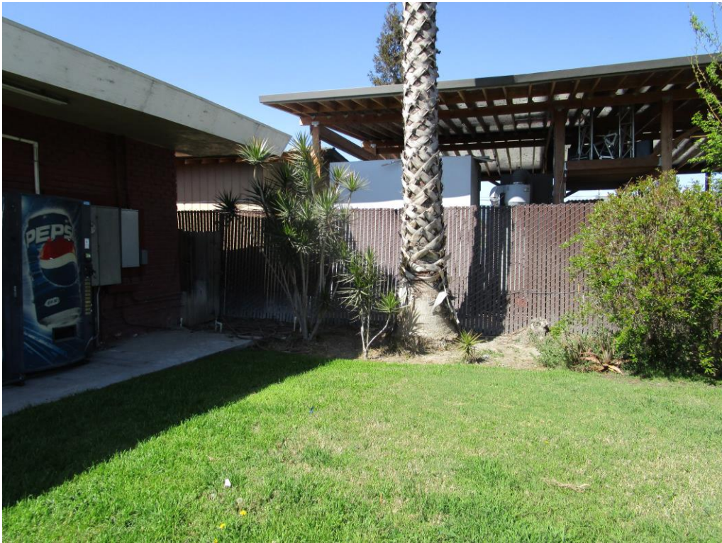
Photo 19: View of electrical panels on rooms along the northwestern portion of subject property.
