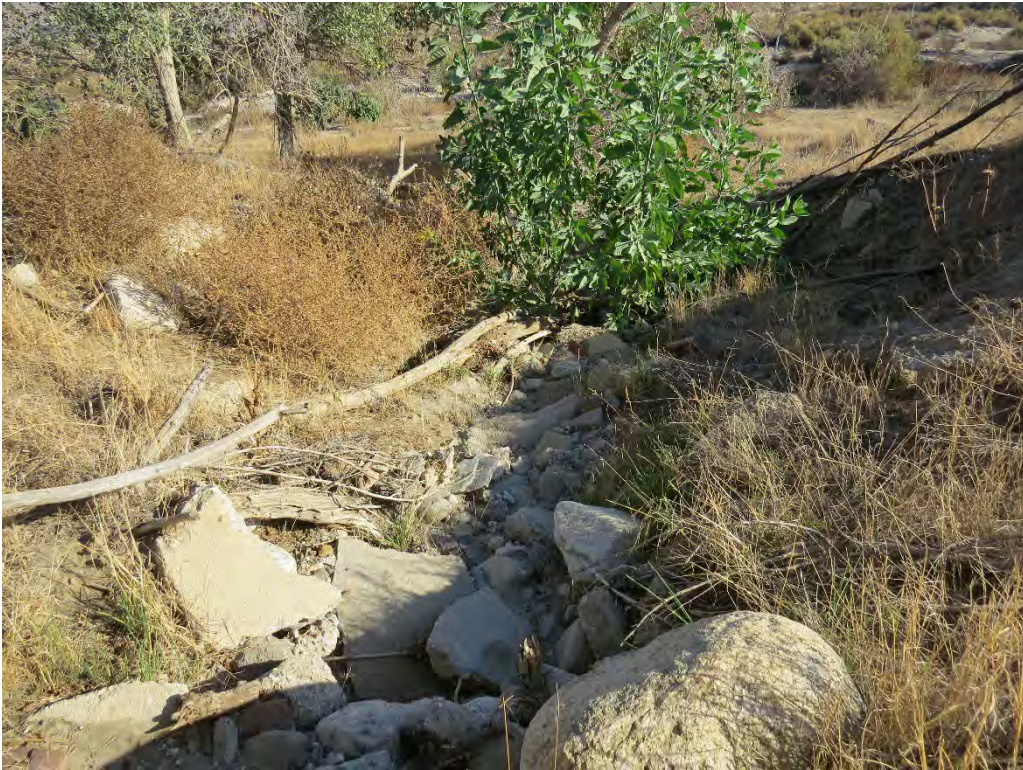
Photograph 4: Concrete debris in the swale associated with the roadside ditch onsite.
