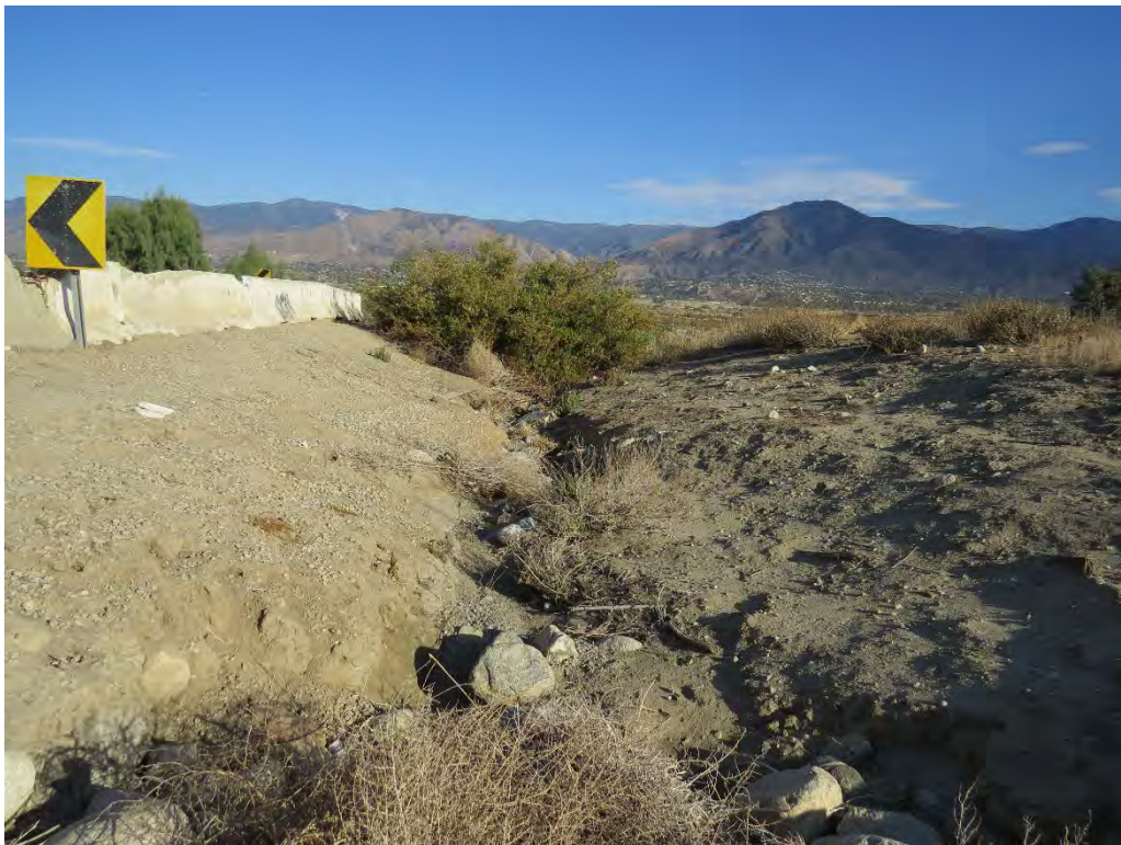
Photograph 2: Looking at the discharge point of the roadside ditch, just outside of the project footprint near the southwest corner of the site on the bluff above the Santa Ana River.
