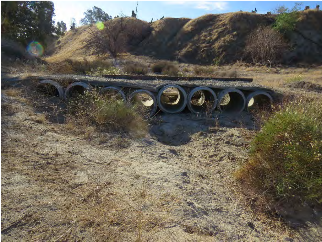
Photograph 11: Small bridge in the middle of Drainage 1 that conveys flows via several culverts.
