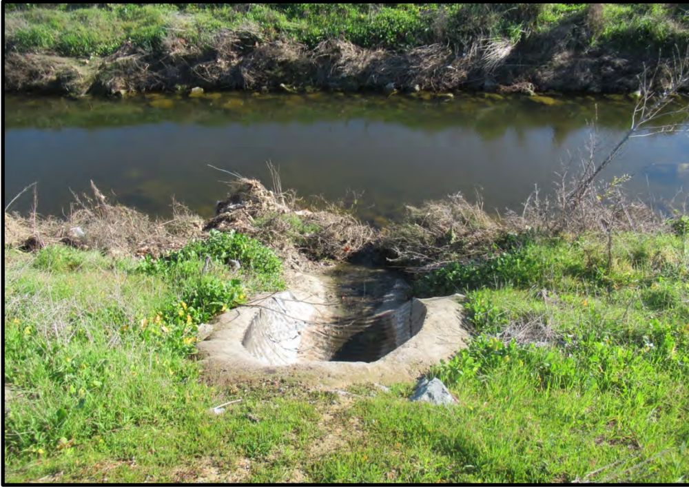
Storm drain outfall structure in Marsh Creek, looking northeast; 01/25/22. The proposed subdivision will tie into this stormdrain system, which extends underground through the center of the site.
