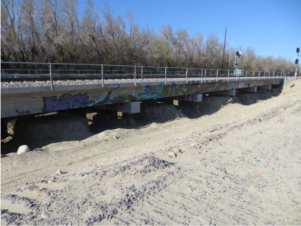
Photograph 7: A photograph of the railroad bridge located within the northern portion of the action area, facing southwest.
