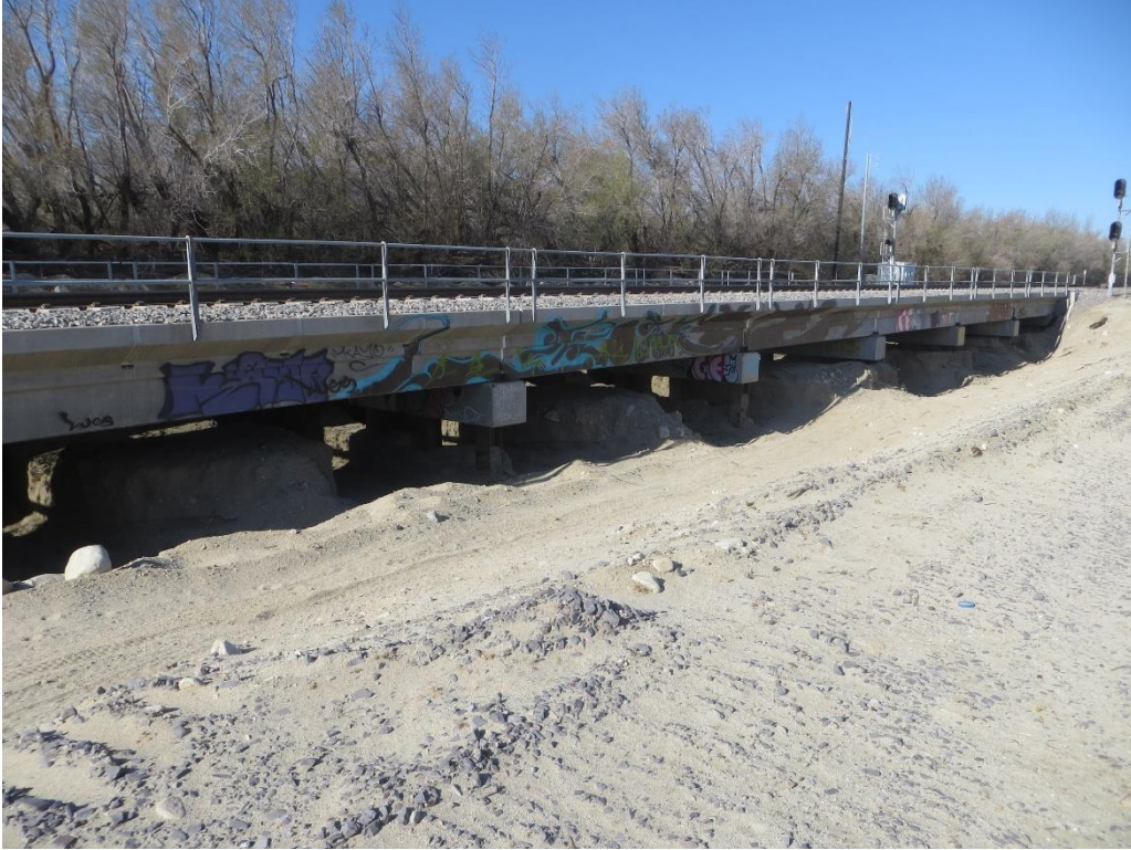
Photograph 7: A photograph of the railroad bridge located within the northern portion of the action area, facing southwest.
