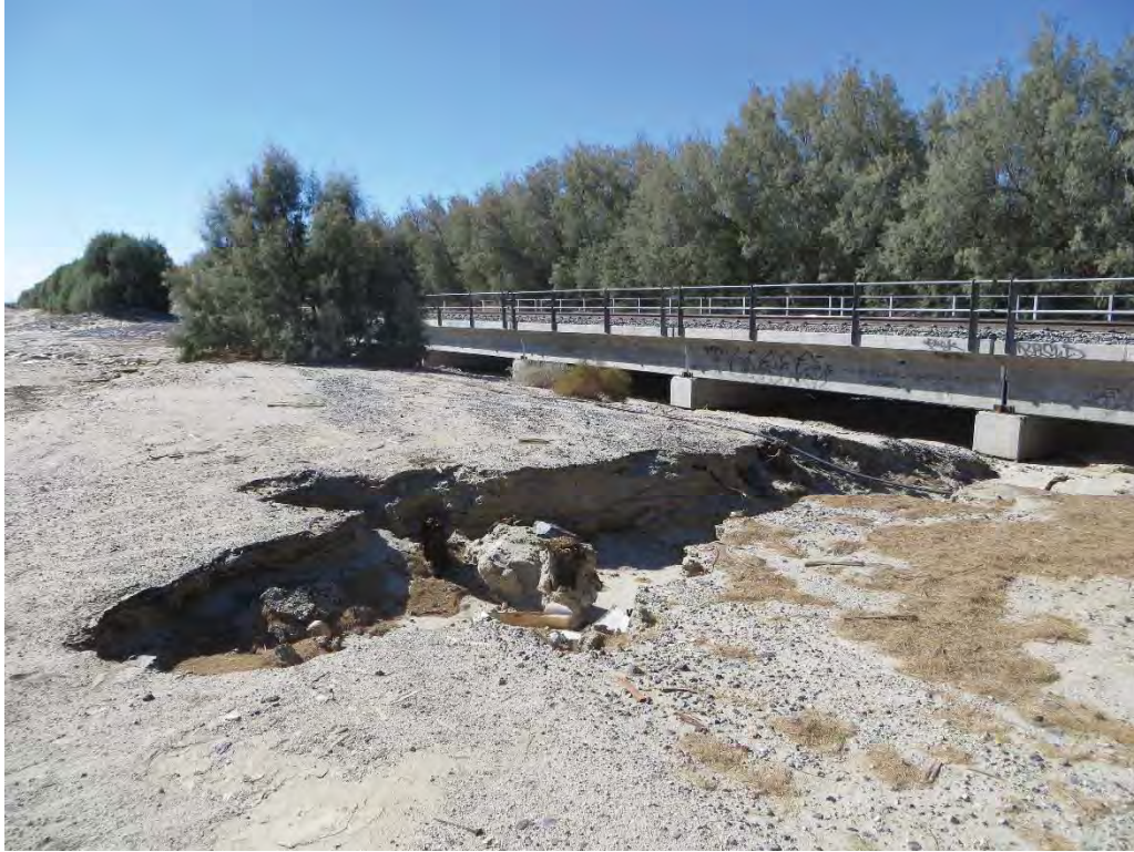
Photograph 7: Facing southeast. The project would utilize this bridge undercrossing to allow the movement of water from the north to the south from the Morongo Wash to the Whitewater River.
