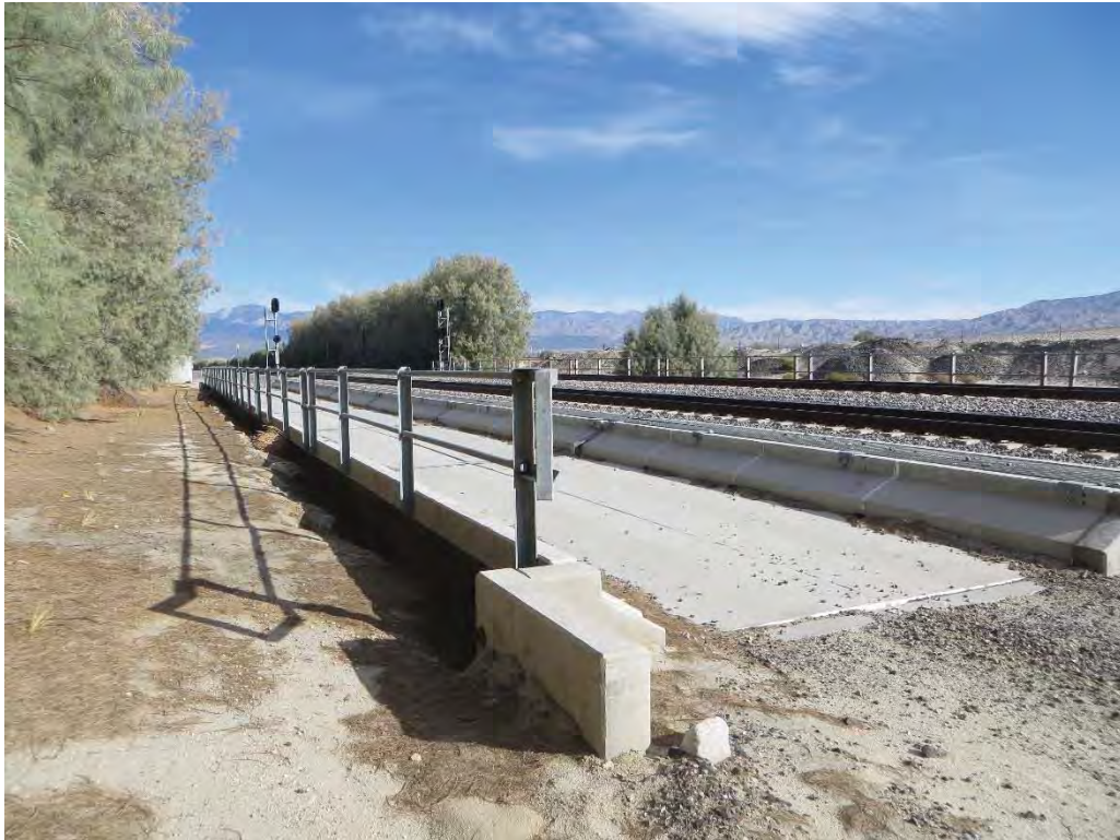
Photograph 6: Facing northwest. The project would utilize this bridge undercrossing to allow the movement of water from the north to the south from the Morongo Wash to the Whitewater River.
