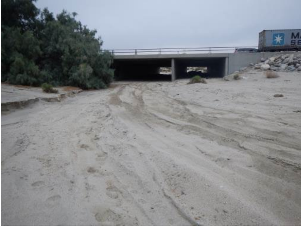
Photograph 29 – Looking northeast (upstream) at the southern end of the Reach 3 I-10 crossing.
