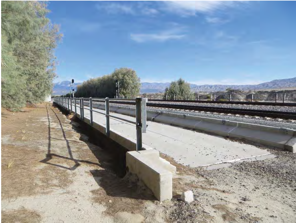
Photograph 6: Facing northwest. The project would utilize this bridge undercrossing to allow the movement of water from the north to the south from the Morongo Wash to the Whitewater River.
