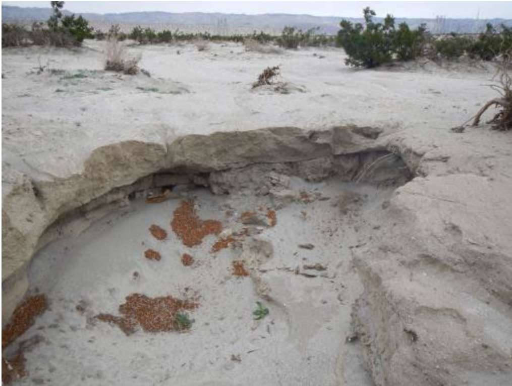
Photograph 9 – Looking northeast (upstream) at a newly developed headcut area, showing a clear demarcation between the upland and the watercourse within Reach 3.
