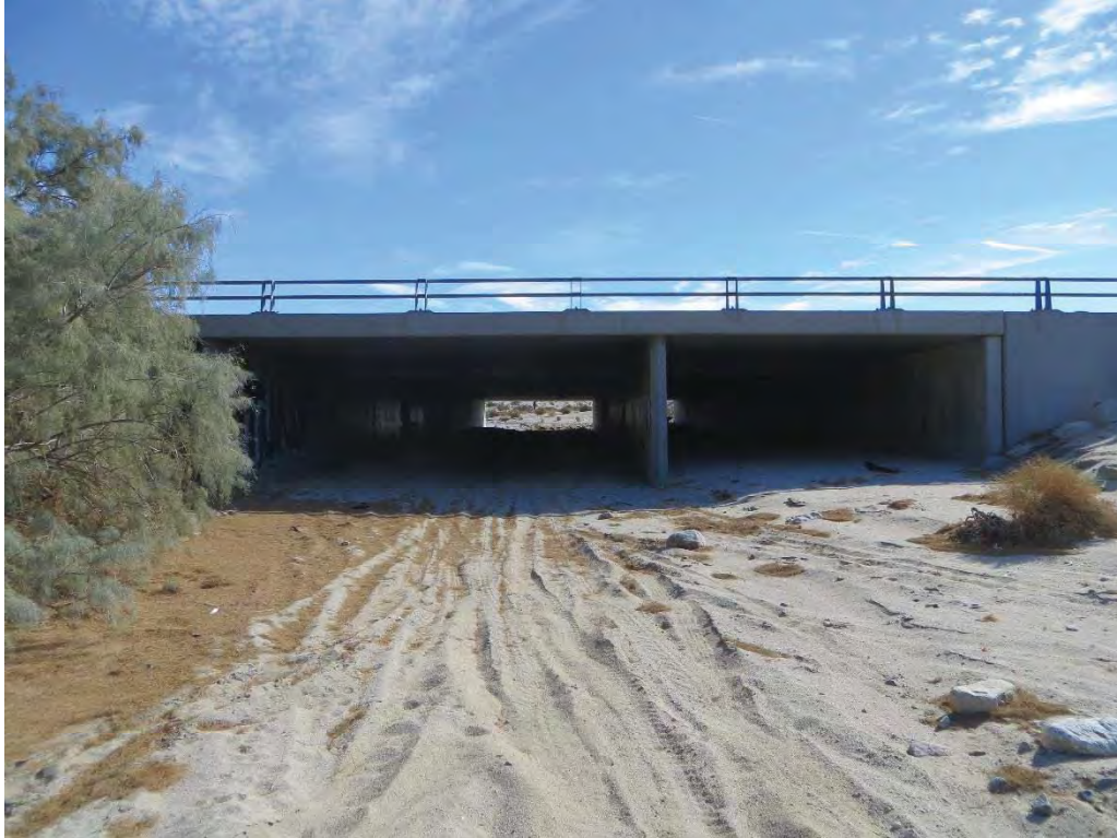
Photograph 9: Facing north. This crossing allows movement of wildlife, water, and sand under Interstate 10. However, because of the windrows and railroad tracks, water is currently restricted once it enters the area between the interstate and railroad tracks.
