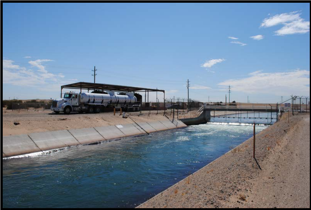
Figure A1. Chlorination Dosing Station at Drop One (Tanker offloading Chlorine)
