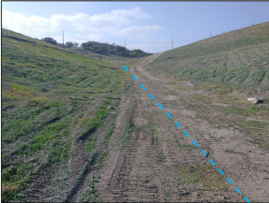
Photo 3. View west of the drainage showing lack of definition due to historical and ongoing land use. Approximate path of the drainage shown in blue (12-08-21).
