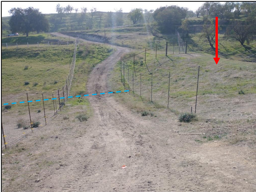
Photo 4. View south of dirt access road crossing the drainage (dashed blue line). Note the earthen berm (red arrow) just upstream of the property impounding the drainage (12-08-21).
