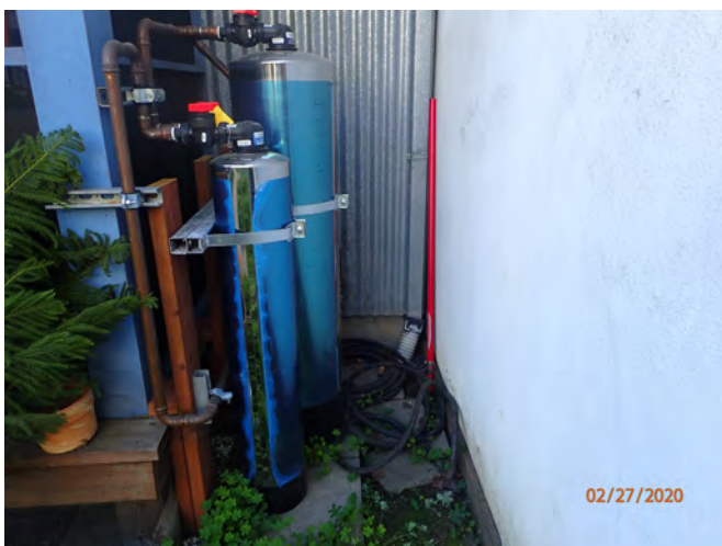
Photo 11: Fluoride treatment/removal tanks at southwest corner of residence.
