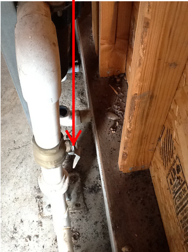
Irrigation Shut Off Valve
