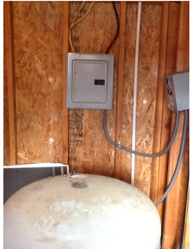
Electrical Sub Panel
