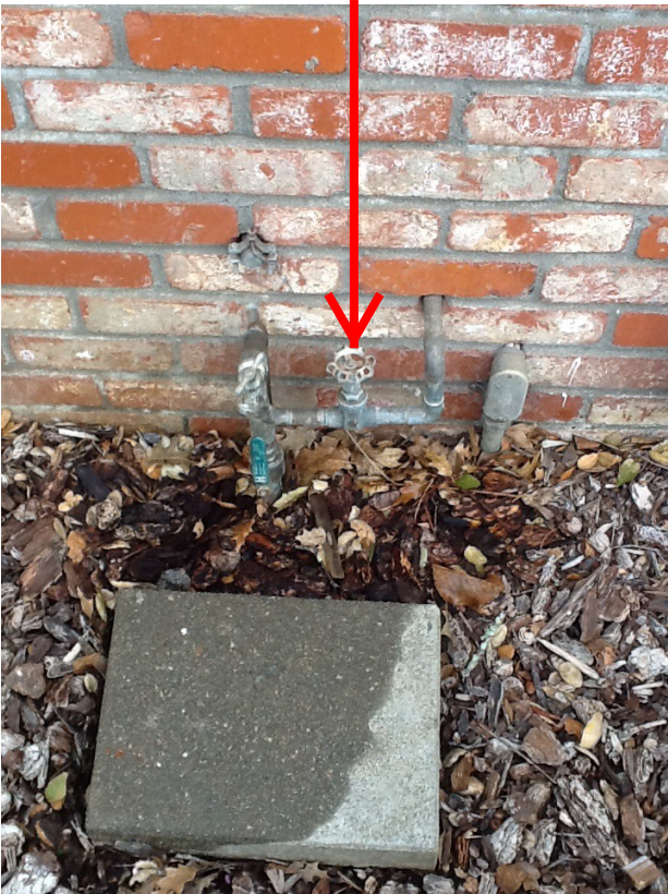
House Shut Off Valve
