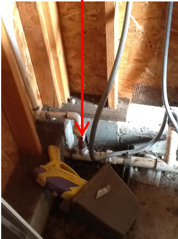
Pool Fill Shut Off Valve
