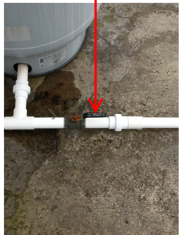
Main Shut Off Valve
