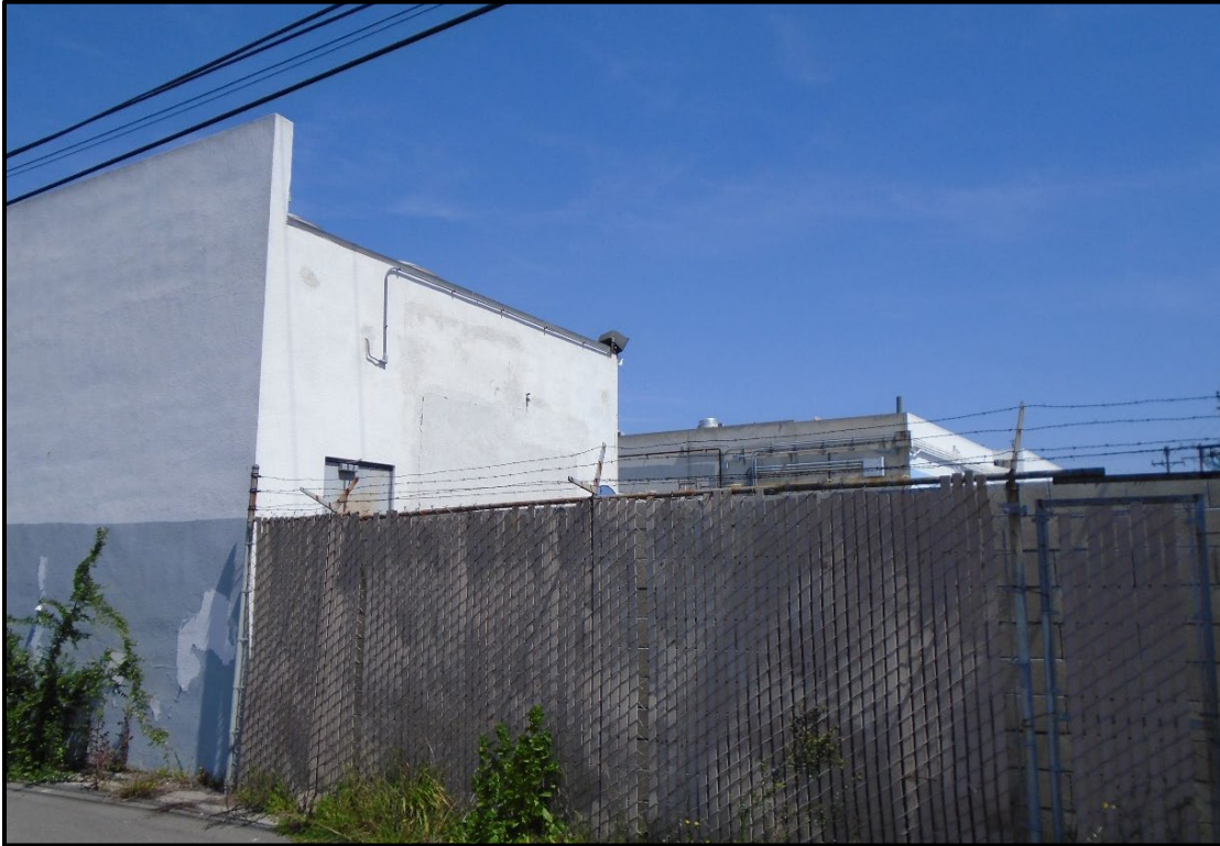
Figure 26. Building 4 (16907 South Normandie Ave., APN 6106-030-017), partial view of south elevation, view northeast
