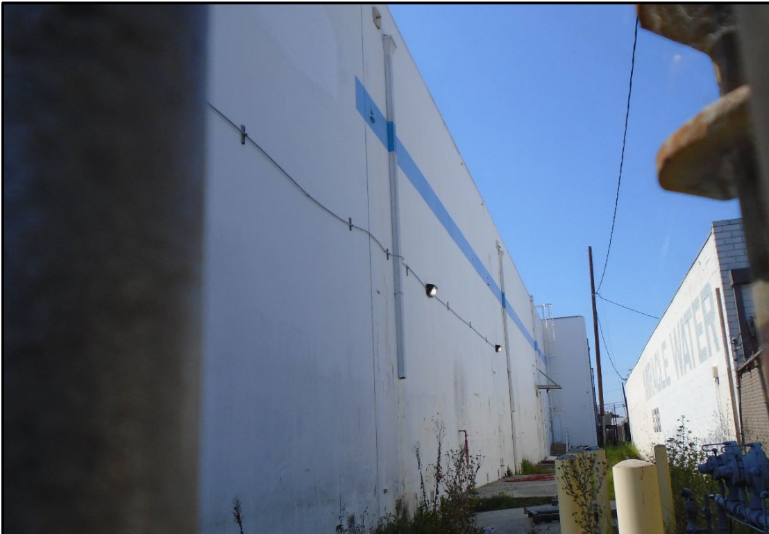
Figure 29. Building 4 eastern addition (16907 South Normandie Ave., APN 6106-030-017), partial view of north elevation, view southwest
