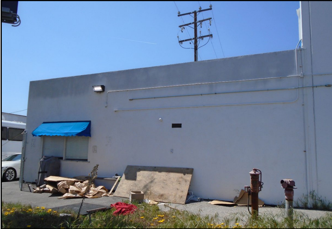
Figure 28. Building 4 eastern addition (16907 South Normandie Ave., APN 6106-030-017), partial view of east elevation, view southwest
