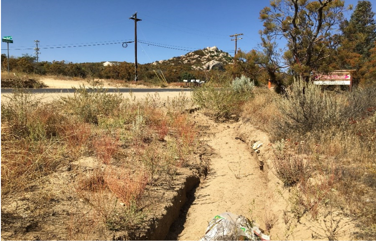
Photograph 5. Bautista substation and erosional feature created from sheet flow off of Bautista Road in the distance, facing northwest.
