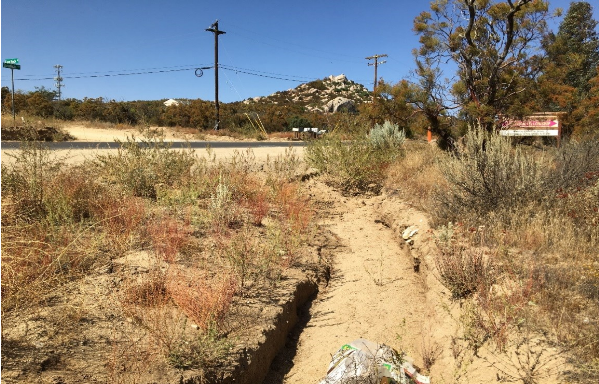
Photograph 5. Bautista substation and erosional feature created from sheet flow off of Bautista Road in the distance, facing northwest.
