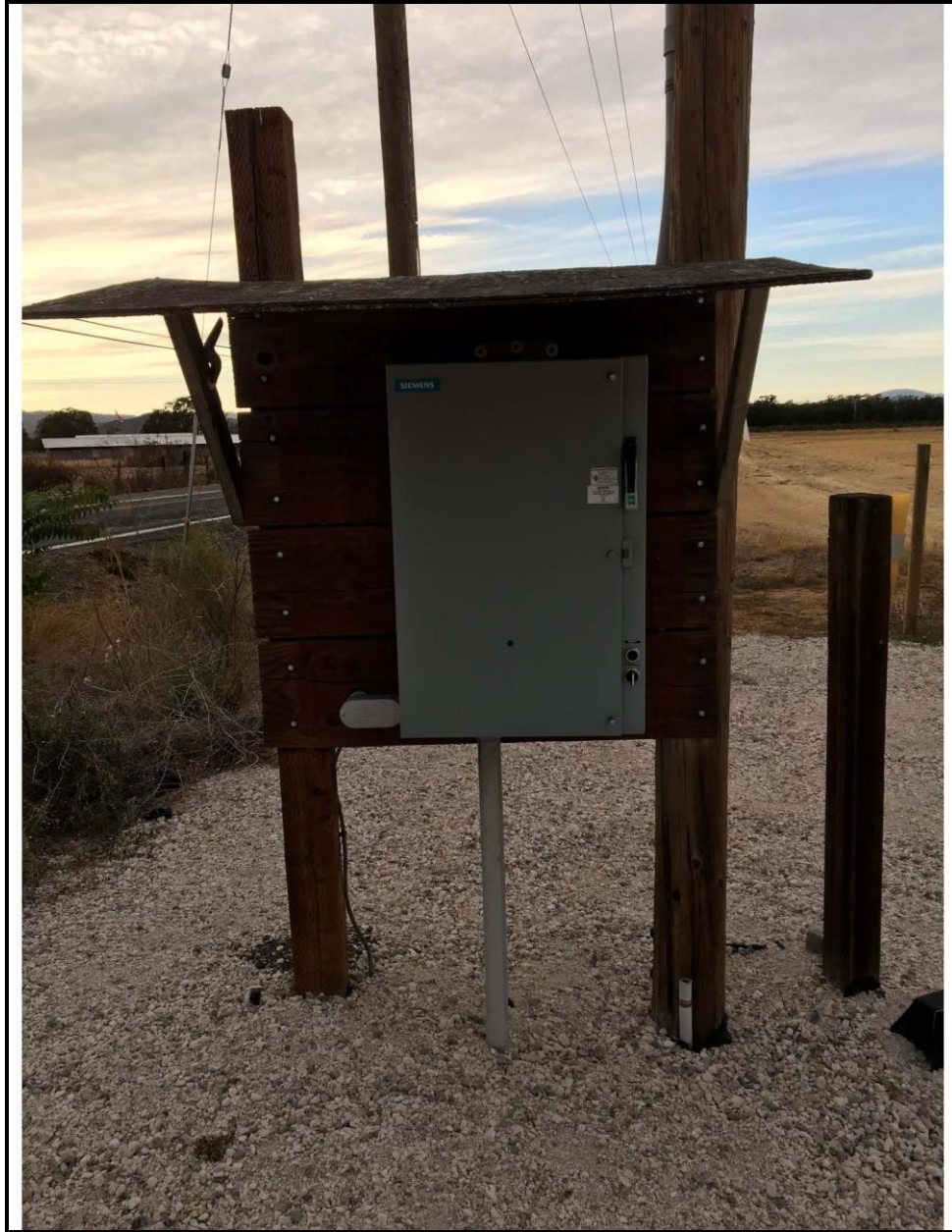
Photo 1: View control Panel for project Irrigation Well.
