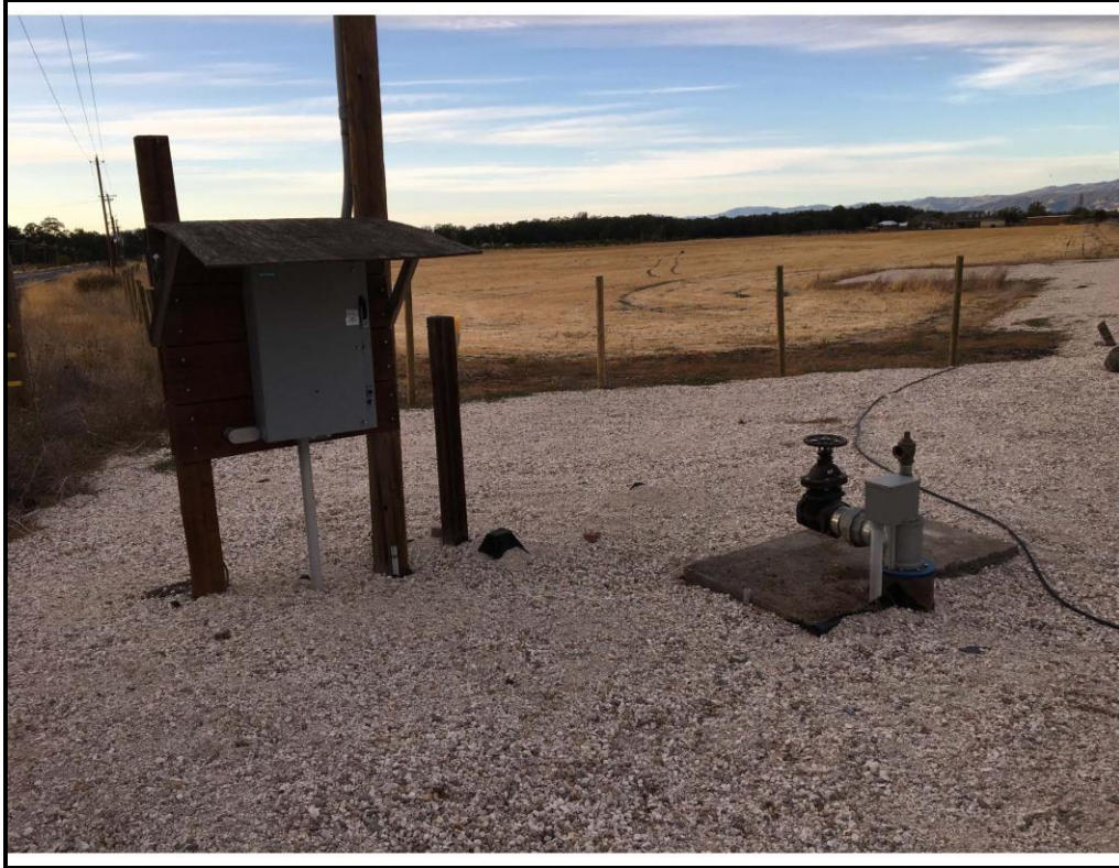
Photo 3: View of project Irrigation Well and Control Box located at southeast corner of the Site.
