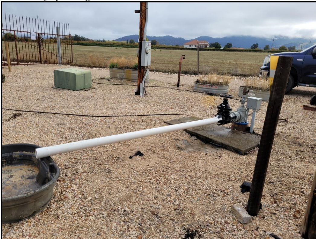
Photo 4: View of Irrigation Well during the Nov. 2, 2021 Test w/ 4-inch diameter discharge pipe
