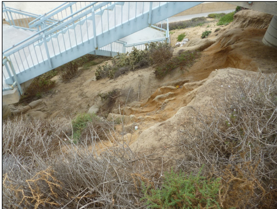
Photo 4. Erosion and erosion control materials (left) underneath one of the stairways.
