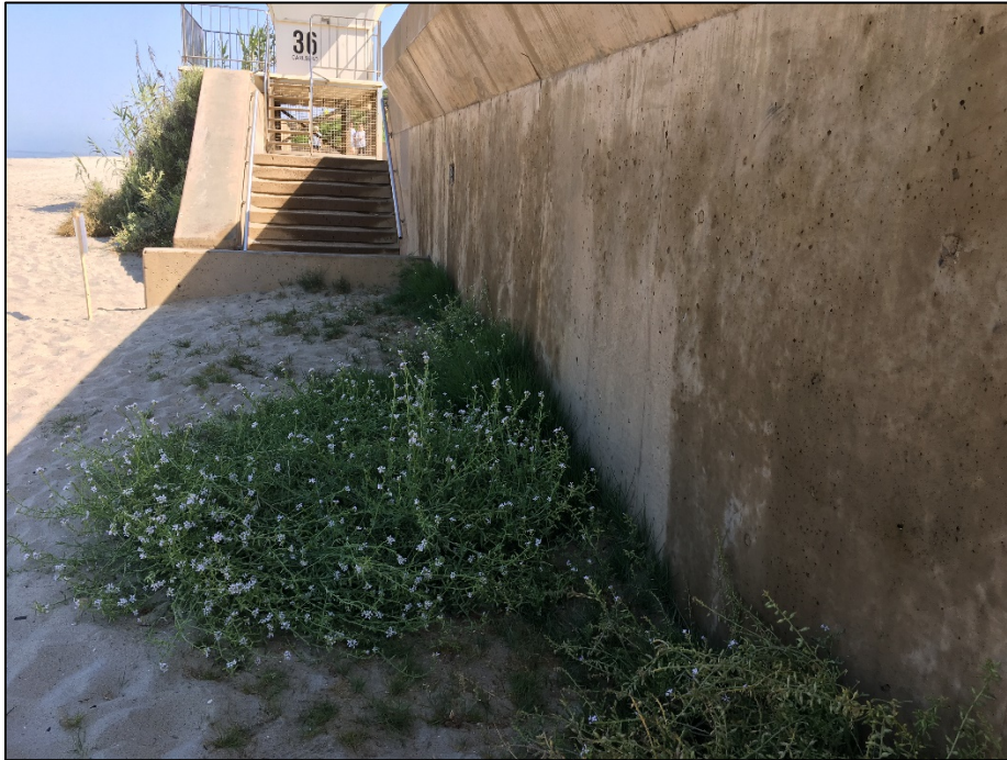
Photo 7. View of western side of sea wall and native and nonnative vegetation growing in sandy soils. A portion of sandbar willows and Arundo can be seen in the background. Date: June 3, 2020.
