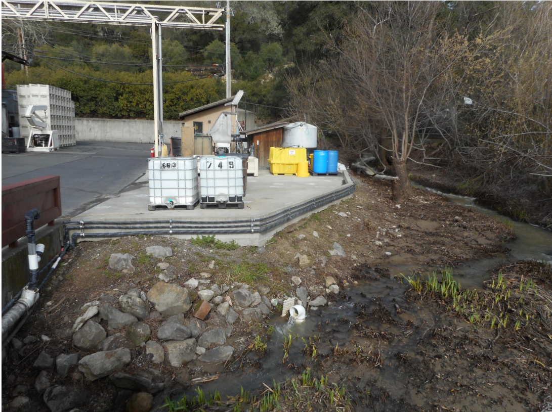
Figure 2. Unpermitted pad adjacent to permitted structures, that is proposed to remain within the Stream Setback Zone.
