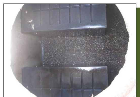
Fully cleaned separation chamber.
