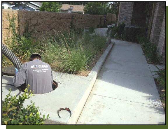
Vacuuming out of media filters.
