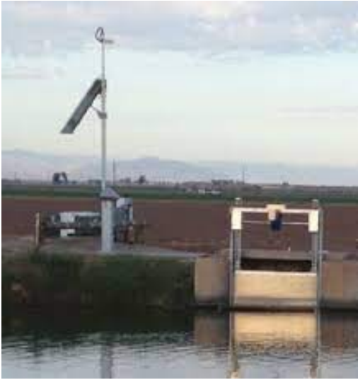
Typical Rubicon Slip Gate with Solar and SCADA Antenna
