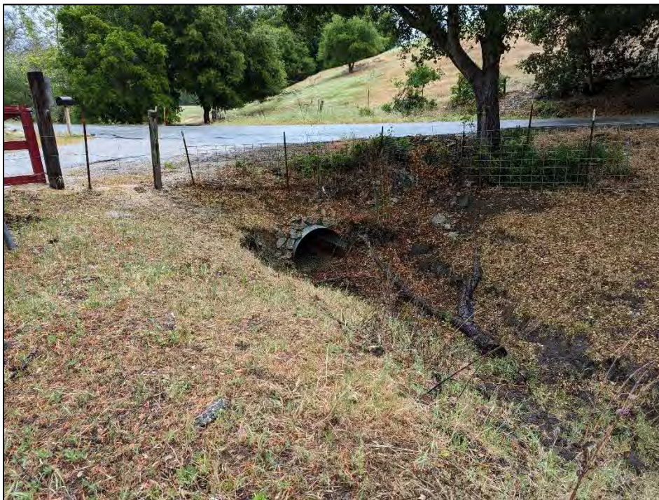
Photo 4. View north of the culvert outlet at Monte Road and the existing driveway (April 21, 2022)
