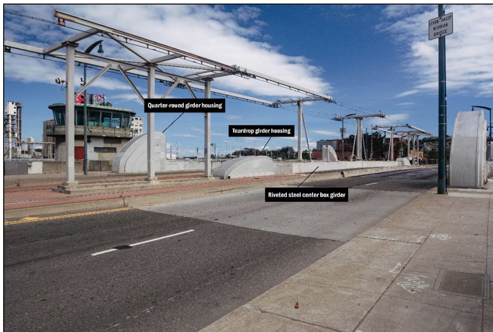
Photograph 1. Above-deck character-defining features including quarter-round and teardrop girder housing units with Art Moderne styling and riveted steel center box girder, facing southeast
