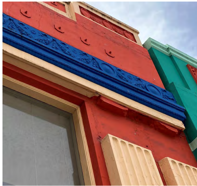
Figure 46: Detail of garland ornamentation and missing capitals above the west pair of pilasters.
