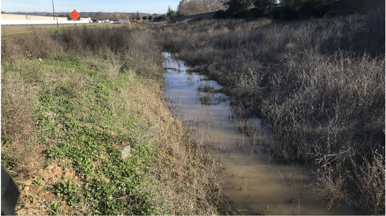
Photograph 7: View of eastern drainage with standing water south of McBean Park Drive. 38.88894444 N°, -121.27633333 W° facing east. Photograph taken by Sarah Yates on February 4, 2021.
