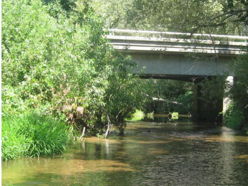
Photograph 9: Facing upstream of the McBean Park Drive Bridge. Photograph taken August 15, 2014 by A. Rich.
