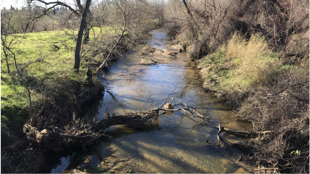
Photograph 3: View of the southern portion of Auburn Ravine from the McBean Park Drive bridge. 38.89018888 N°, -121.28303611 W° facing south, southwest. Photograph taken by Lisa Sandoval on February 5, 2021.
