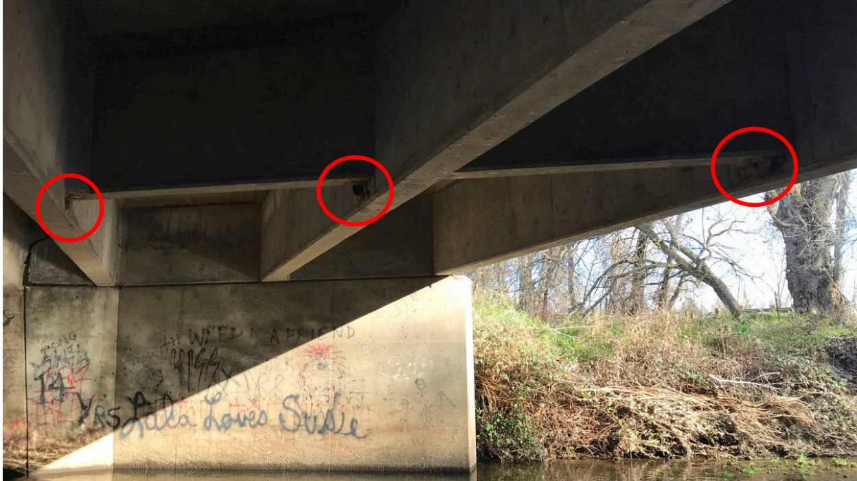
Photograph 17: View of remnant swallow mud nests (in red) on the underside of the bridge over the main channel. 38.890331 N°, -121.283007 W° facing east. Photograph taken by Danielle Temple on February 4, 2021.
