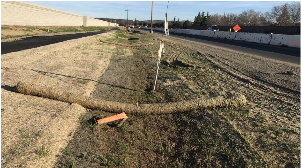
Photograph 8: View of eastern drainage with erosion control measures north of McBean Park Drive. 38.88920833 N°, -121.27616388 W° facing east. Photograph taken by Sarah Yates on February 4, 2021.
