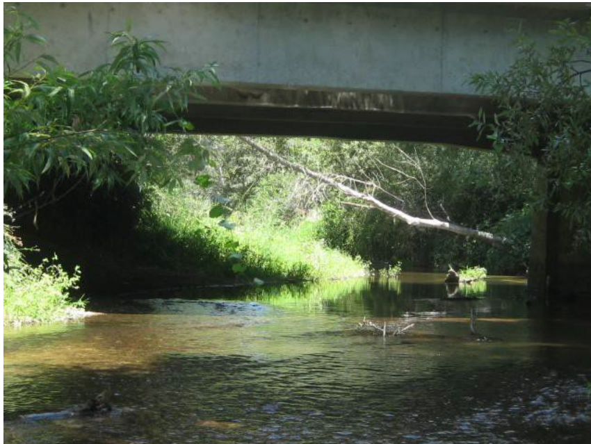
Photograph 10: Facing upstream of the McBean Park Drive Bridge. Photograph taken August 15, 2014 by A. Rich.
