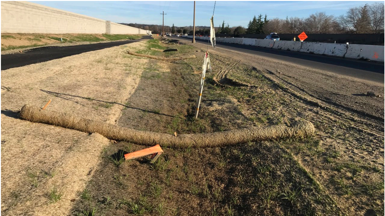
Photograph 8: View of eastern drainage with erosion control measures north of McBean Park Drive. 38.88920833 N°, -121.27616388 W° facing east. Photograph taken by Sarah Yates on February 4, 2021.
