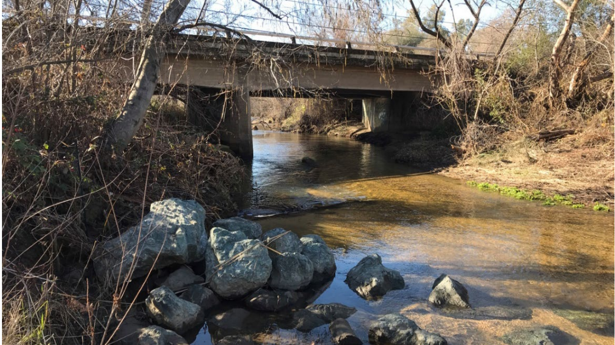
Photograph 1: View of the northside of the existing McBean Park Drive Bridge. 38.89046111 N°, -121.28284444 W° facing south, southwest. Photograph taken by Julie Hausknecht on February 5, 2021.
