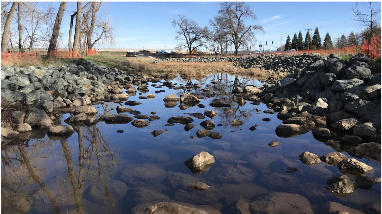
Photograph 6: View of the wetland restoration project north of McBean Park Drive, east of Auburn Ravine. 38.89051944 N°, -121.28282777 W° facing east. Photograph taken by Julie Hausknecht on February 4, 2021.
