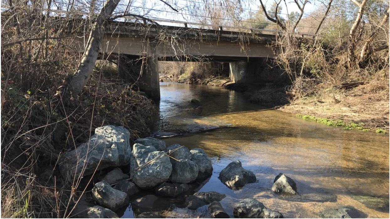
Photograph 1: View of the northside of the existing McBean Park Drive bridge. 38.89046111 N°, -121.28284444 W° facing south, southwest. Photograph taken by Julie Hausknecht on February 5, 2021.
