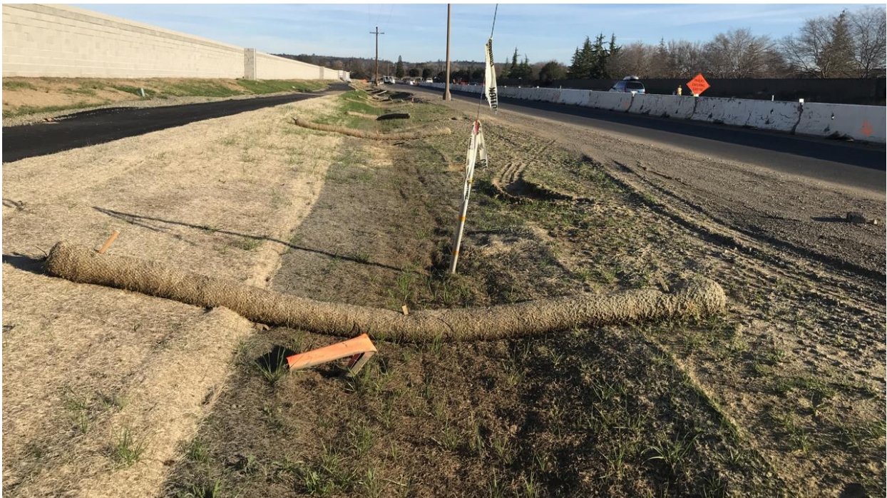
Photograph 8: View of eastern drainage ditch (Ditch 1) with erosion control measures north of McBean Park Drive. 38.88920833 N°, -121.27616388 W° facing east. Photograph taken by Sarah Yates on February 4, 2021.
