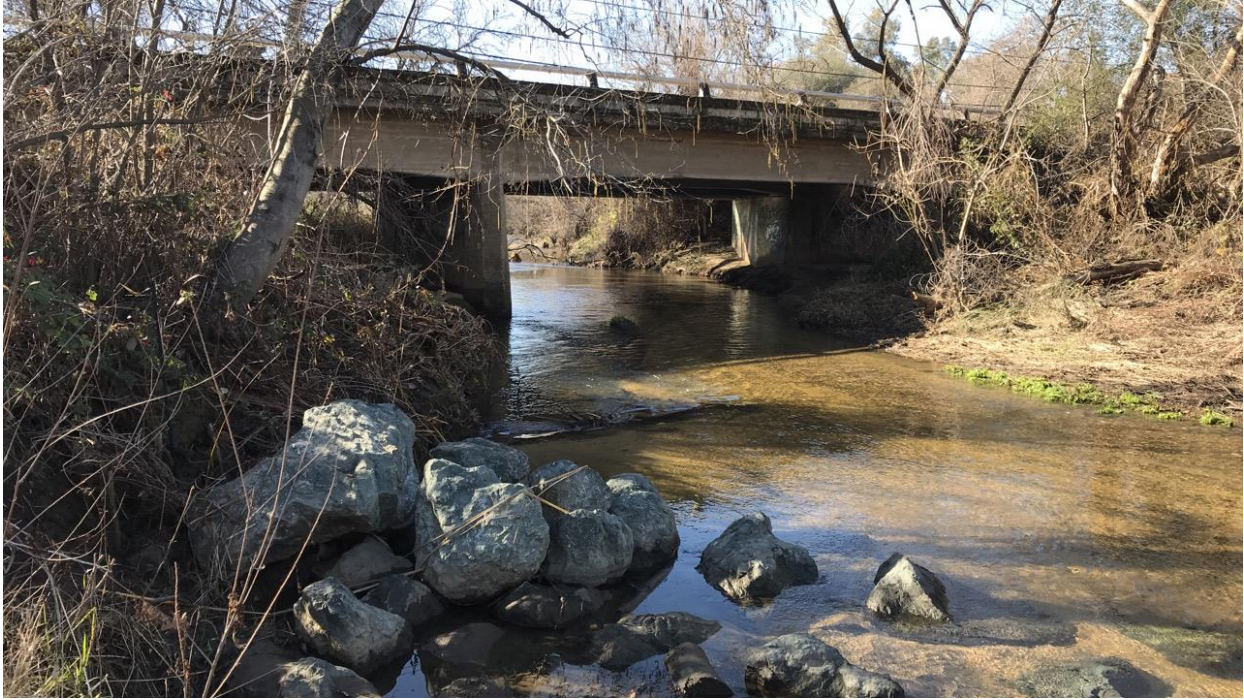
Photograph 1: View of the northside of the existing McBean Park Drive Bridge. 38.89046111 N°, -121.28284444 W° facing south, southwest. Photograph taken by Julie Hausknecht on February 5, 2021.
