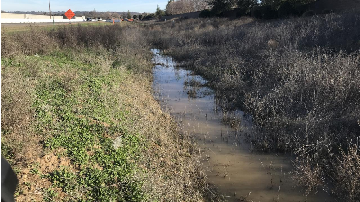
Photograph 7: View of eastern drainage ditch (Ditch 2) with standing water south of McBean Park Drive. 38.88894444 N°, -121.27633333 W° facing east. Photograph taken by Sarah Yates on February 4, 2021.
