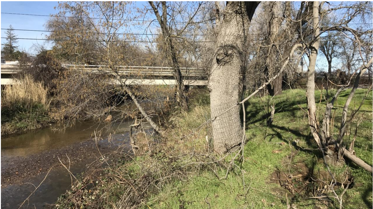
Photograph 2: View of the southside of the existing McBean Park Drive Bridge. 38.889821 N°, -121.283272 W° facing north. Photograph taken by Julie Hausknecht on February 4, 2021.
