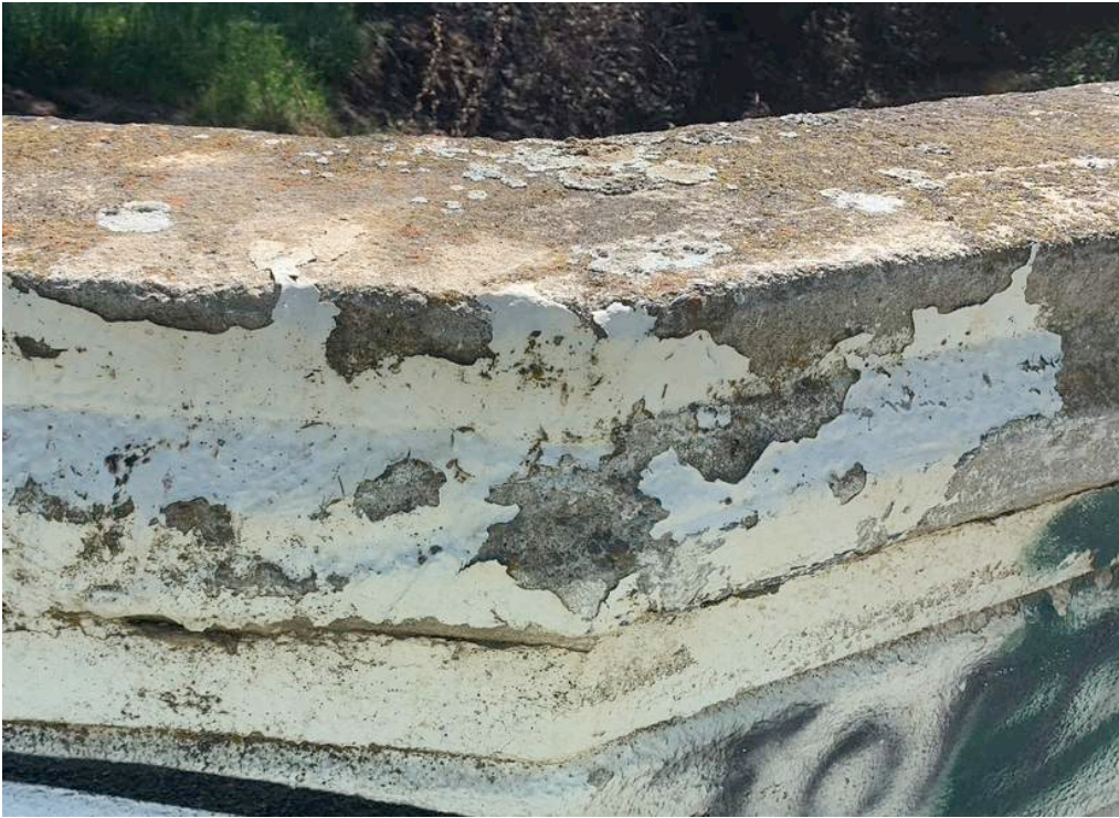
Photo 3. Flaking and peeling paint at northeast corner.
