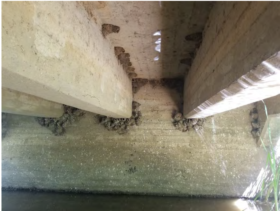
Overview of the under side of the Union School Slough Bridge where evidence of past cliff swallow ( Petrochelidon pyrrhonota ) nesting were observed during the June 23, 2020 field visit. Taken facing north.
