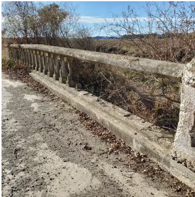
Figure 6. Bridge damage, viewing southwest
