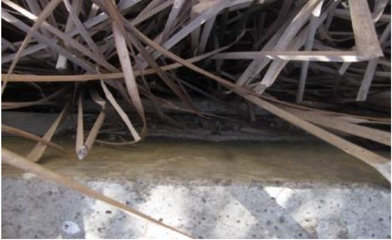
Photo 5 Water gate enabling periodic flow from dredge disposal ponds to freshwater marsh FM-04 (12/14/19)
