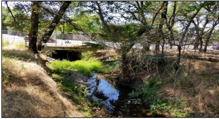
Photo Point 1. View of Verde Cruz Creek – Intermittent Channel, downstream view towards Manzanita Avenue (facing northwest). Taken on May 10, 2018.
