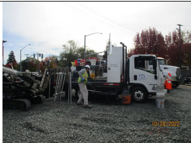
Steam cleaning equipment
