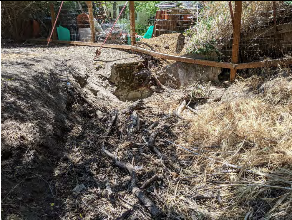
5. Facing west, photo shows a view of where the drainage leaves the Property via a partially obstructed culvert that diverts flows beneath the adjacent property. Photo taken July 12, 2021.
