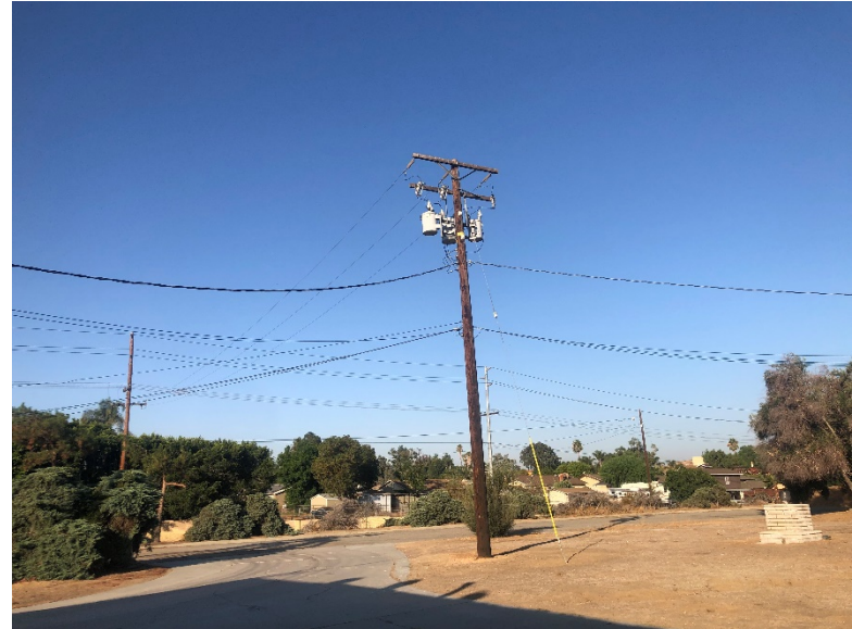
Photo 14: Power pole w/transformer Dairy access road
