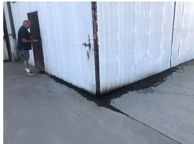
Photo 12: Oil seepage from East end Dairy shed
