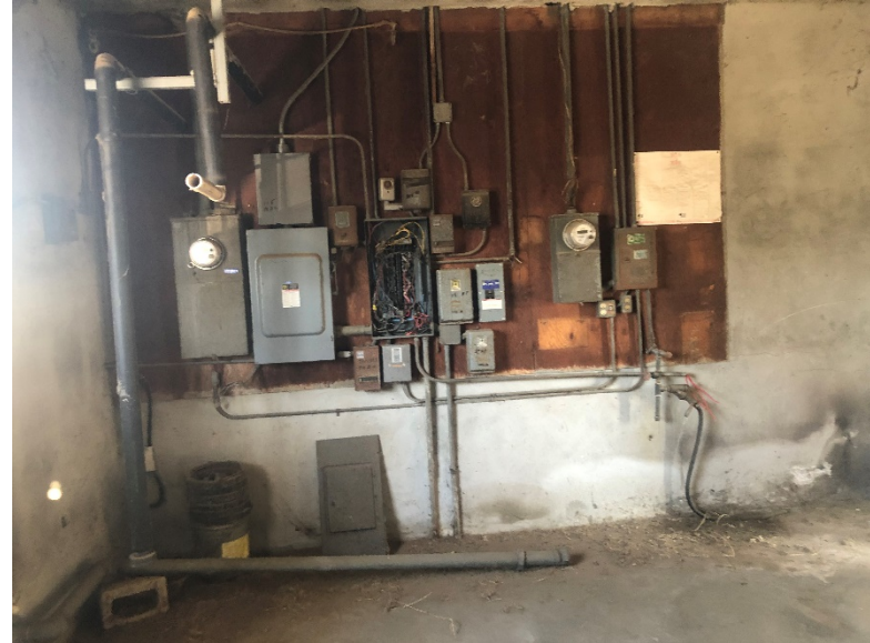
Photo 6: Dairy Building electrical room
