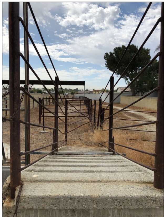
Detail view of concrete cattle loading chute located behind the main residence.
