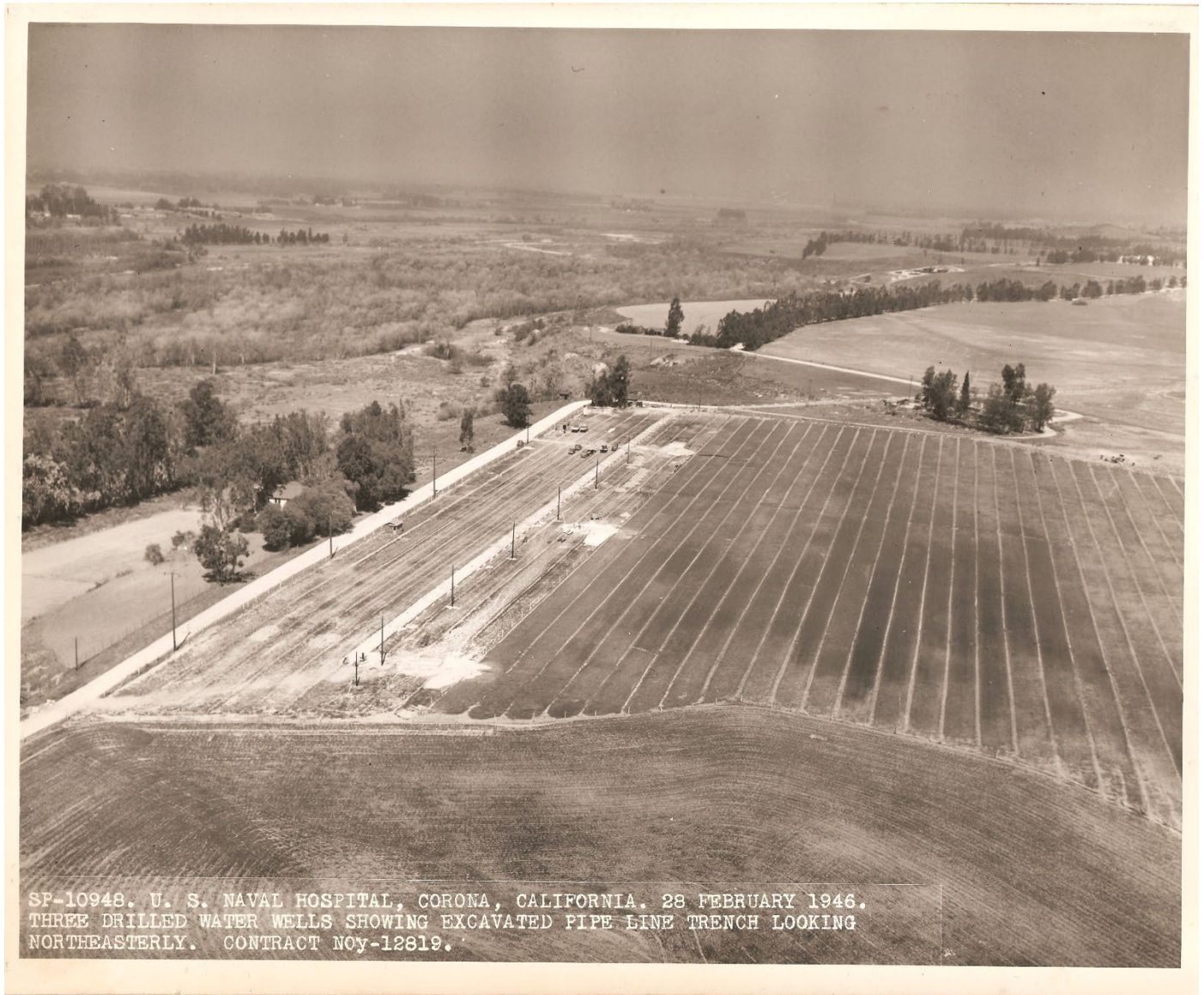
Three drilled water wells showing excavated pipeline trench looking northeasterly. SP-10948; 2-28-1946. Source: Sea Bee Archives, courtesy Kevin Bash.
