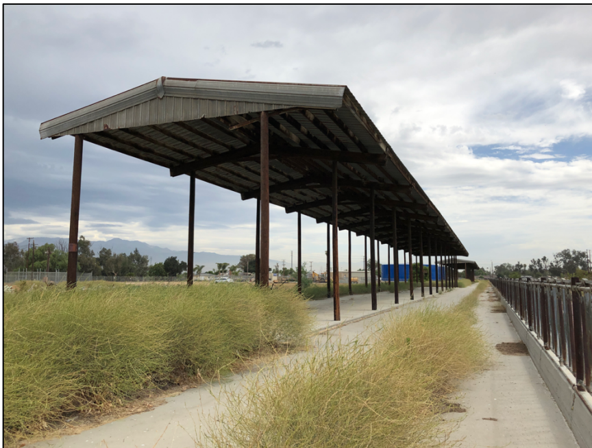
View east of pole structure located behind the main residence. The property has three pole structures that measure over 200-feet in length and one long pole structure that extends over 1,000-feet in length. The pole structures are located directly behind the main residence.
