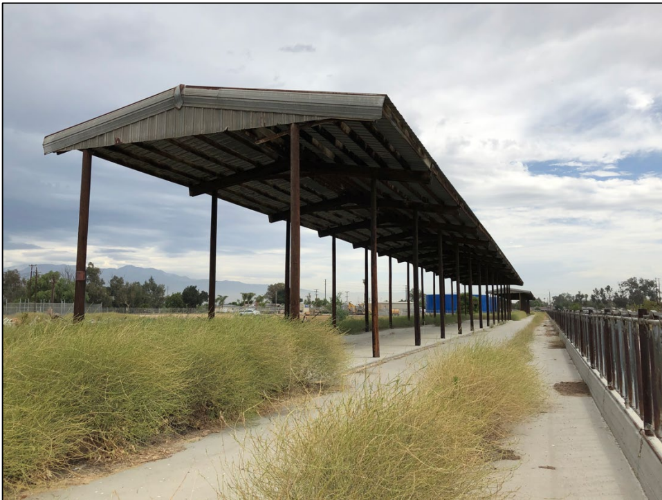
View east of pole structure located behind the main residence. The property has three pole structures that measure over 200-feet in length and one long pole structure that extends over 1,000-feet in length. The pole structures are located directly behind the main residence.
