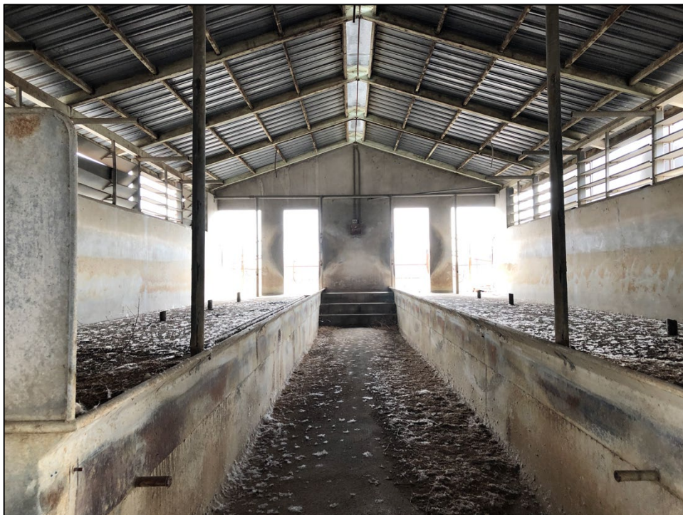
Interior view of the milk parlor's rear section. The milk parlor was constructed in the herringbone style. The herringbone style allowed milkers to more efficiently milk cows without having to kneel because the cows were at an elevated height.
