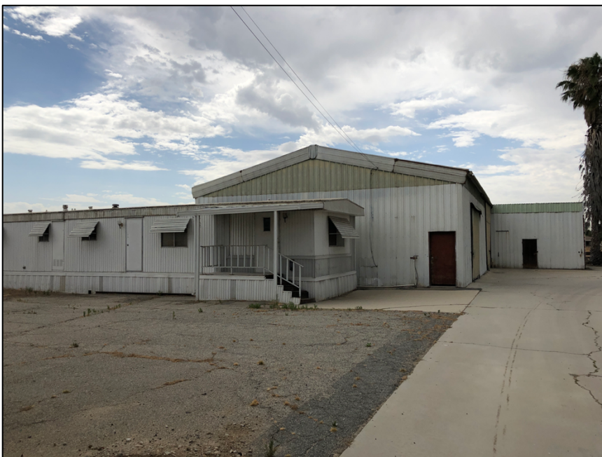
View south of the barn's north elevation. A manufactured trailer is located on the north elevation of the barn and may have served as an additional residence or office.
