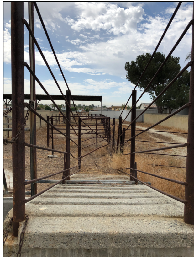
Detail view of concrete cattle loading chute located behind the main residence.
