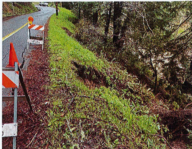
Photo 1. Canyon Road slip-out, facing west (3/23/2023).
