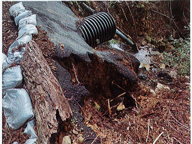
Photo 1. Kings Mountain Road slip-out, facing north (4/11/2023).
