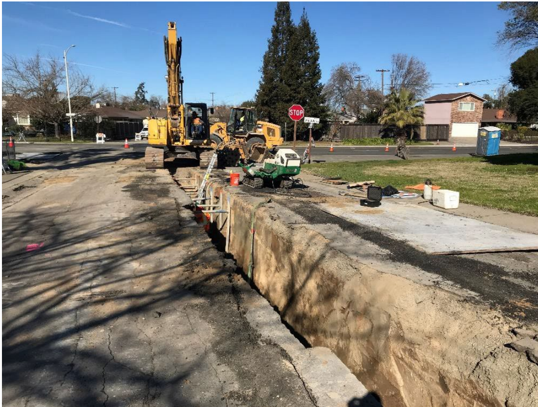
Figure 8. Example of open-cut construction for a 20-inch diameter force main within a paved road.
