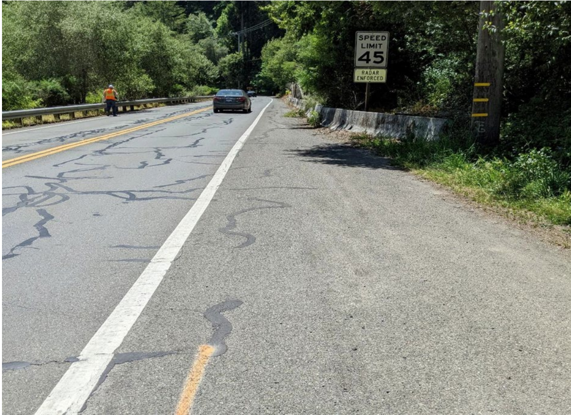
Figure 13. Looking southeast along Highway 116 at the location of the Segment 2 of the Main Force Main pipeline alignment.
