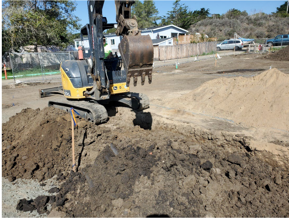
Figure 29: Trenching for utilities on 10/18/22 during the preceding project for the San Simeon Campground Modular at Site 2. Photo by Chad Jackson.
