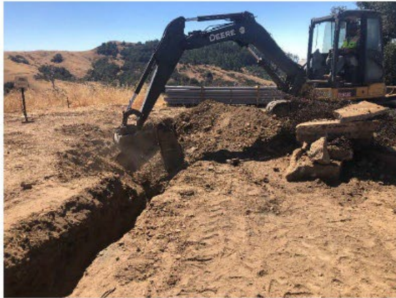
Trenching in the SE corner where the concrete enclosure rubble was unearthed 8/24/23.
