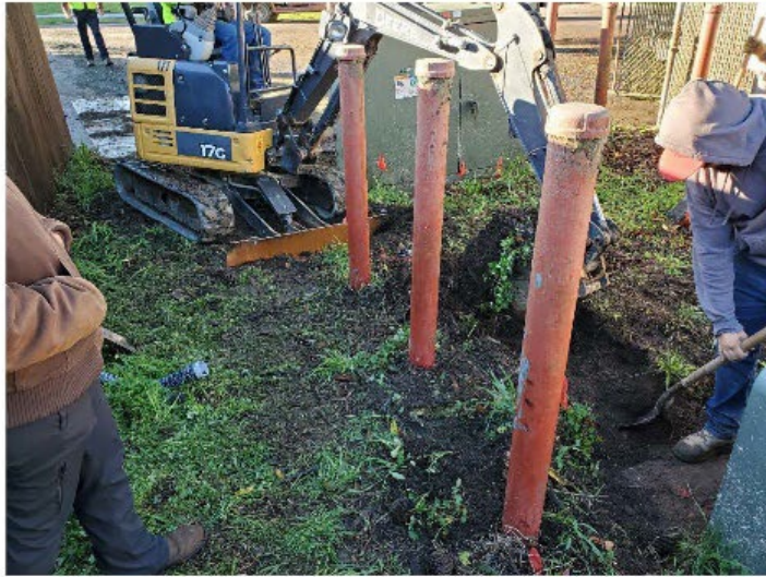
Excavations for electrical utilities showing previously disturbed area at the tie in location to the PGE box. 12/28/23.
