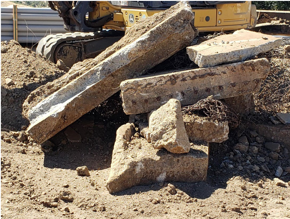
Figure 28: An example of the zoo building remnants uncovered during trenching on Aug. 23, 2022.
