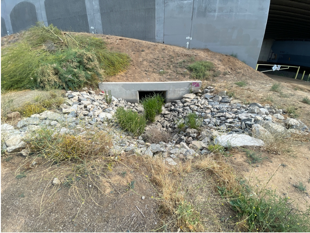
Photo 3. View of northern extent of ephemeral channel and project impacts where storm drain will connect to existing reinforced concrete box culvert, facing north.
