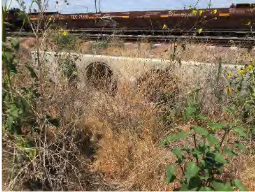
Photo 15. Downstream culverts at the end of F2. The culverts drain across I-215 to a canal within March Air Force Base. Photo taken facing east. July 18, 2018
