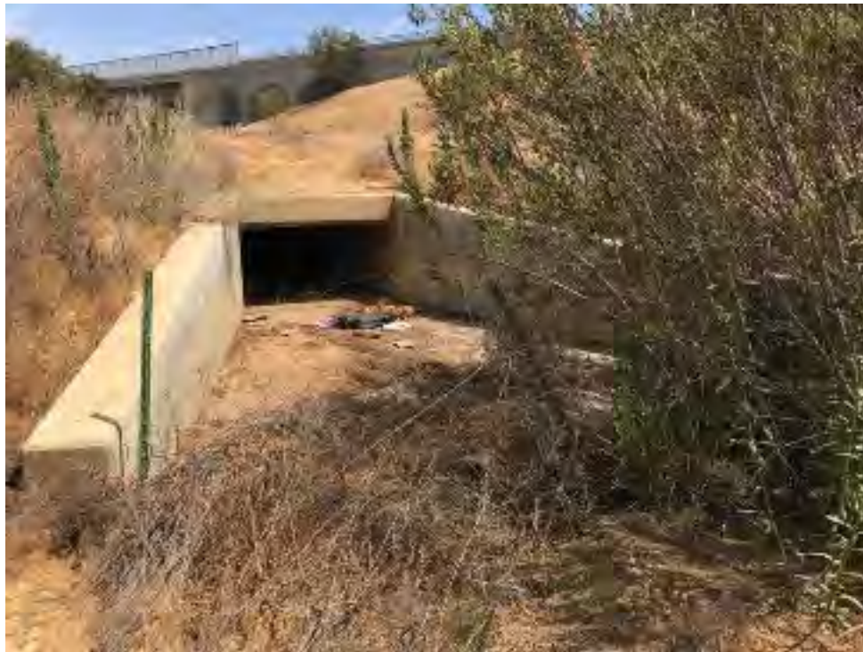
Photo 3. View of F1 downstream culvert. This culvert runs across I-215 to a large canal within March Air Force Base. Photo taken facing south. June 27, 2018
