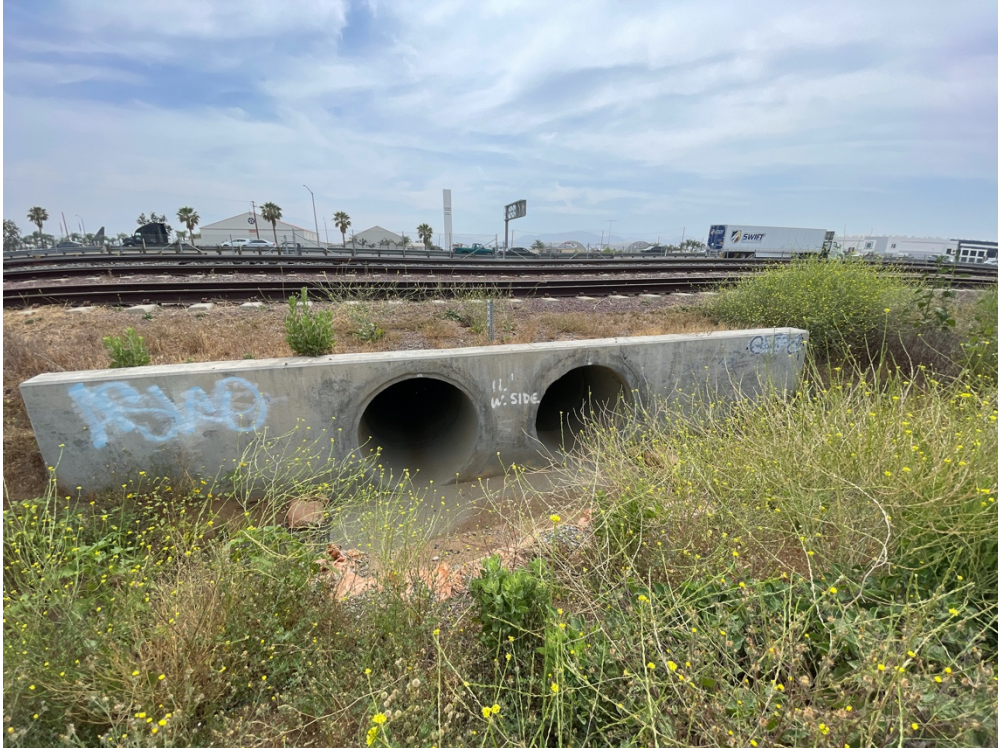
Photo 5. View of dual reinforced concrete box culverts where the storm drain will connect at the southern terminus of the project, facing east.
