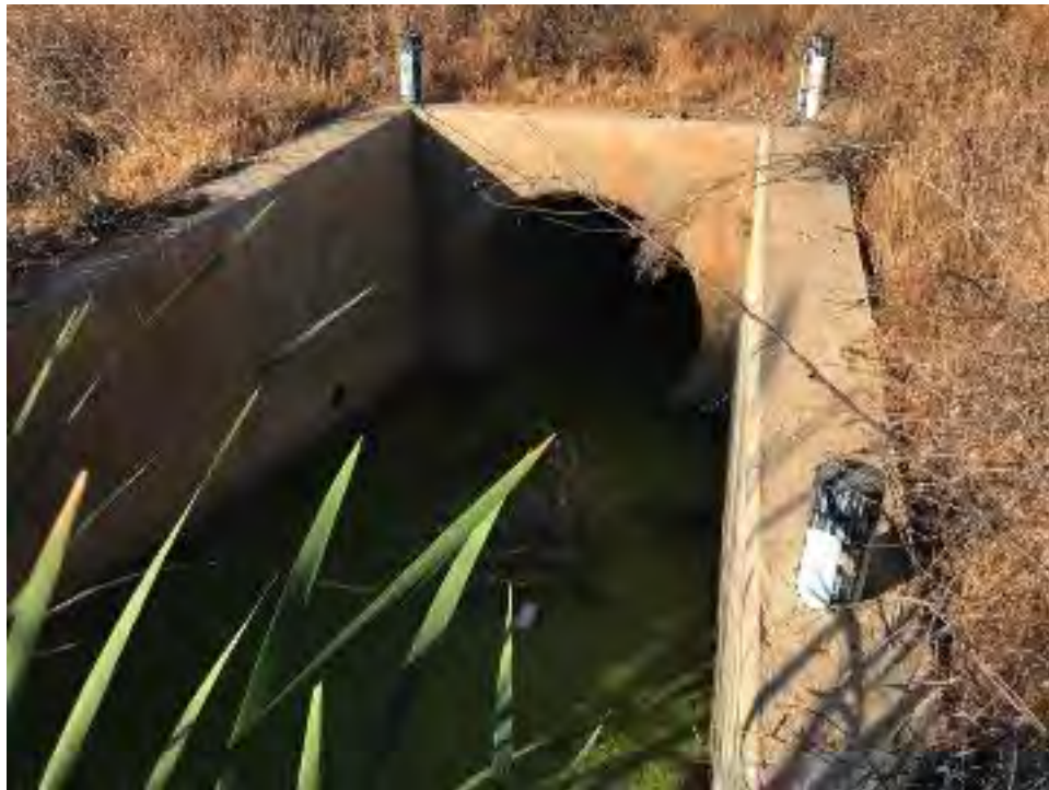
Photo 2. View of one of the culverts that feeds into F1. Culvert contains standing water and is approximately 45 feet away from the culvert that drains the entire feature. June 27, 2018
