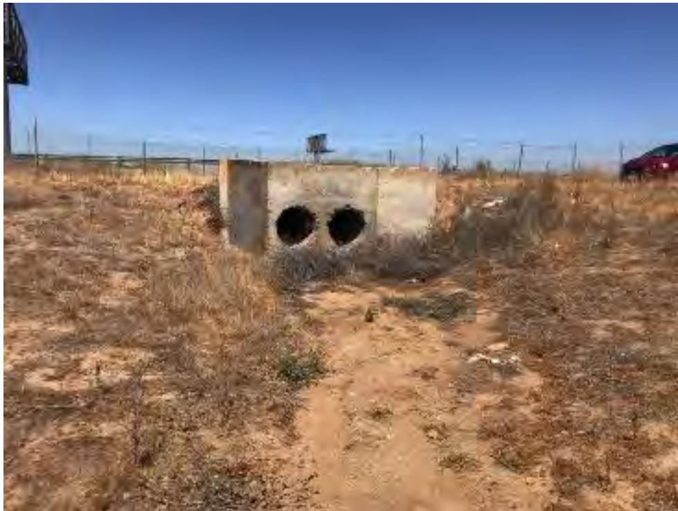
Photo 28. View of additional culvert within March Air Reserve Base. F2 appears to drain across I-215 into this culvert. Photo taken facing west. June 27, 2018
