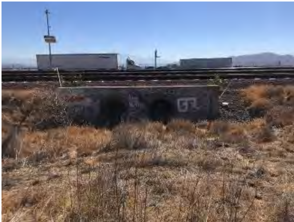
Photo 18. View of F3 downstream culverts. Culverts runs under the railroad track and I-215, draining into a large canal on the adjacent March Air Reserve Base.
