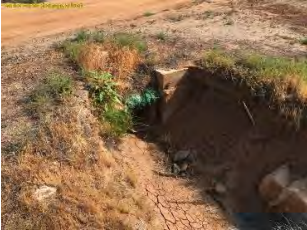
Photo 9. View of a culvert crossing under a dirt road within Feature 2 (F2). Photo taken facing upstream, north. July 18, 2018
