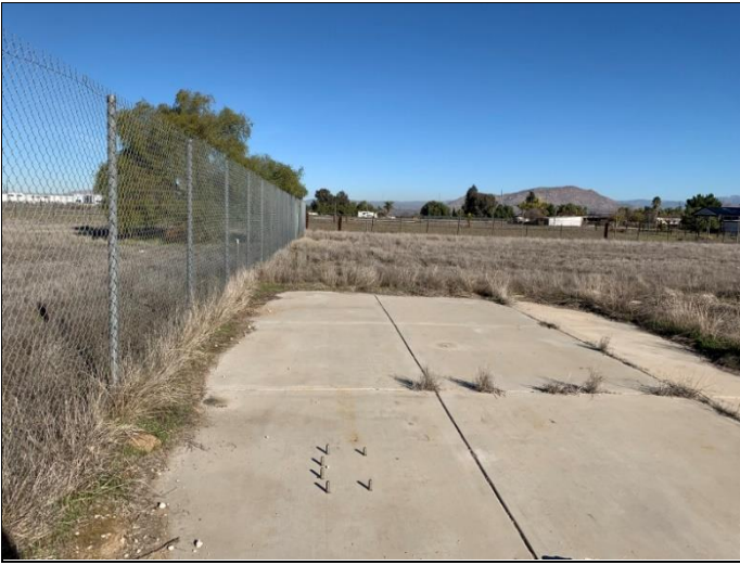
7. Small concrete foundations on the south central portion of the northern parcel, view facing north.
