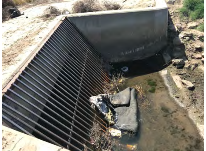
View of existing Peoples Ditch culvert inlet that goes underneath Highway 198, facing south. Visible signs of debris and human disturbance were observed within the canal. April 27, 2020.
