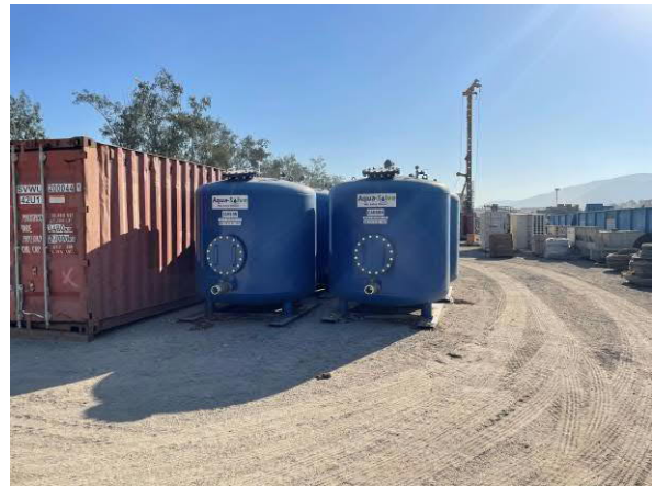
Photo #40 View of water tanks stored on central-southern portion of site.
