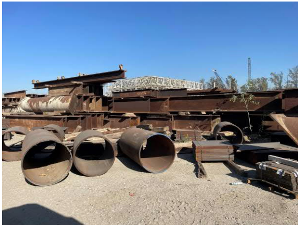
Photo #37 View of loose steel pipe and beam storage on southwestern portion of site.
