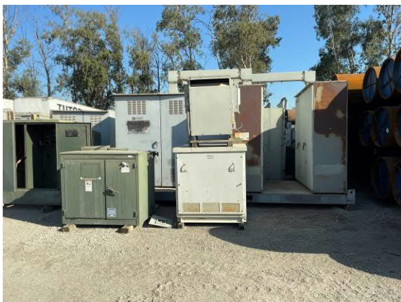
Photo #41 View of transformers (inactive) stored on central portion of site.
