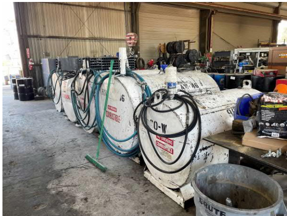
Photo #15 View of oil ASTs in warehouse on central-northern portion of site.
