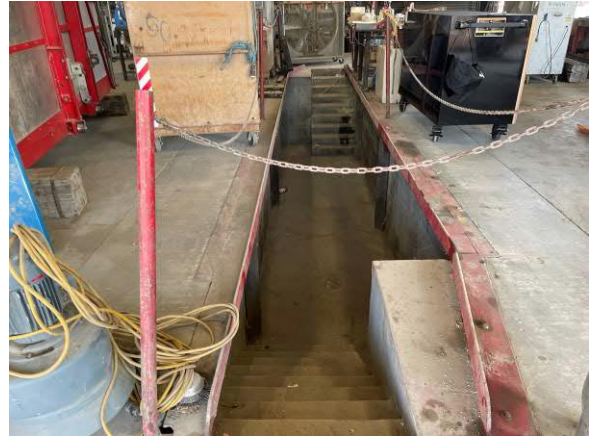
Photo #14 View of former mechanic pit with apparent floor drain located on eastern portion of central-northern warehouse.
