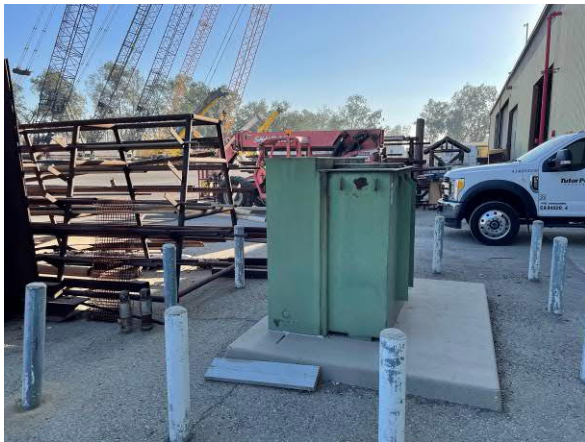
Photo #3 View of pad-mounted transformer on north side of warehouse building, located in central-northern portion of site.
