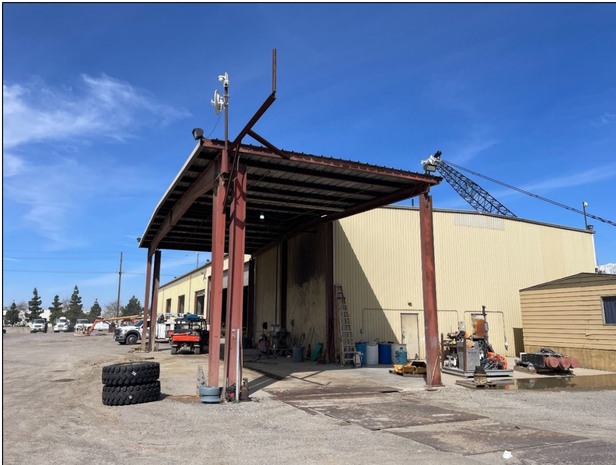
Figure 5-8. Covered work/storage area at southeastern corner of Building 1 at 11171 Cherry Avenue, facing west
