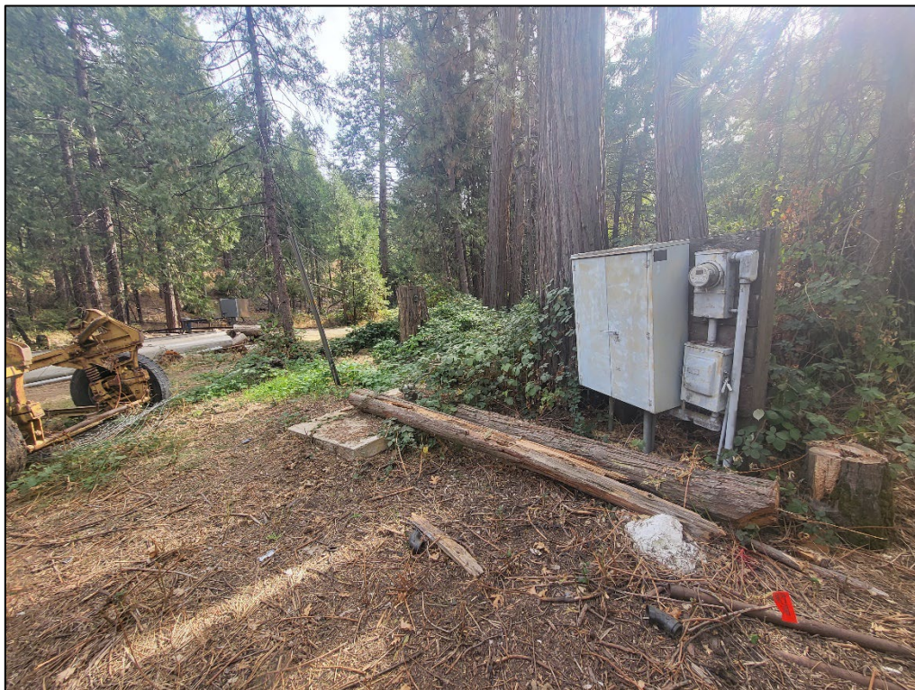
Photo 10. Overview of Well No. 1 (proposed for destruction), with Well No. 4 in background. Surrounded by mixed conifer forest, approximately 75 feet east of Little Fine Gold Creek.
