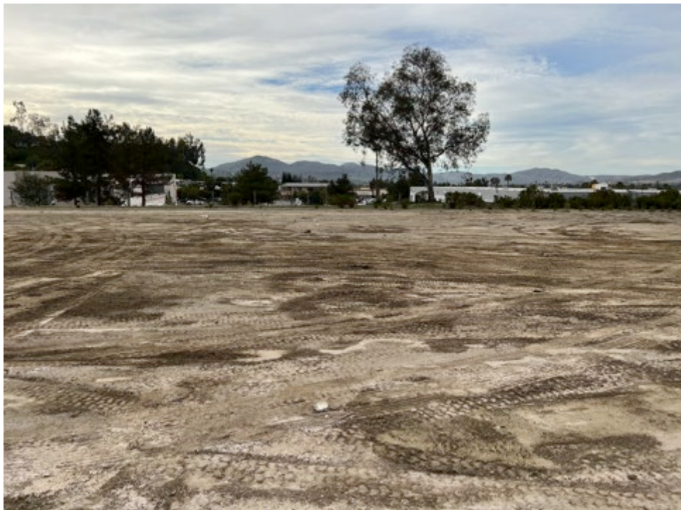
Photograph 4. View of the graded pad in the central portion of the site (Facing west; updated photograph provided by Southwest Signal Service on January 13, 2022).
