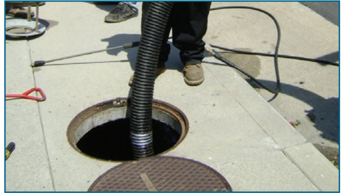
Cleaned easily with vac truck, without catch basin entry, and about 15 minutes is required for service.
