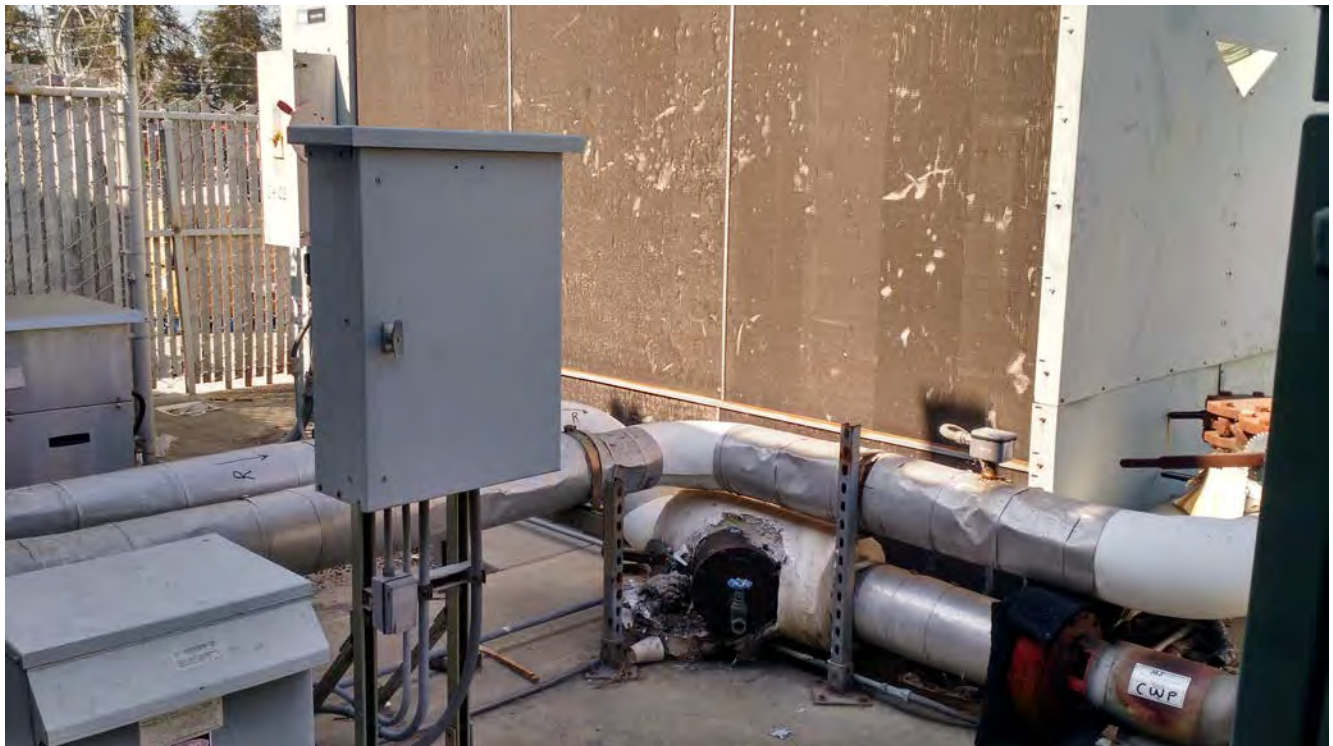
Photo 12: Various machinery and large equipment on the west (back side) of the building – piping, what appears to be a large cooler and electrical equipment.
