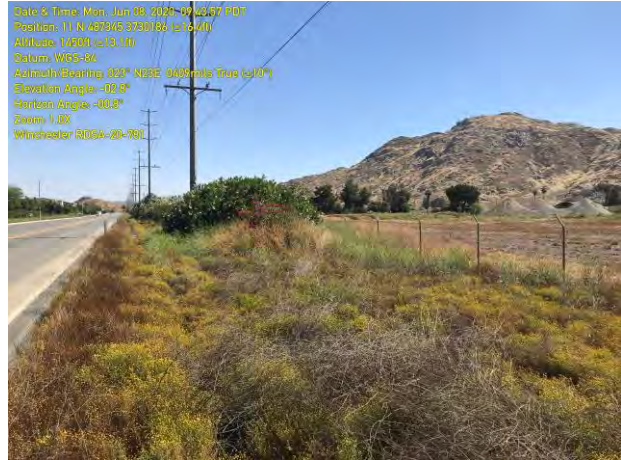
Concrete v-ditch largely obscured by weedy growth, along southwest area of site, facing north. Briggs Road is on the left (06.08.2020).
