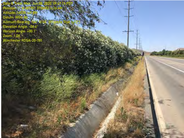
Concrete v-ditch along the west side of the project site, near northwest corner of site, facing south. Briggs Road is on the right (06.08.2020).
