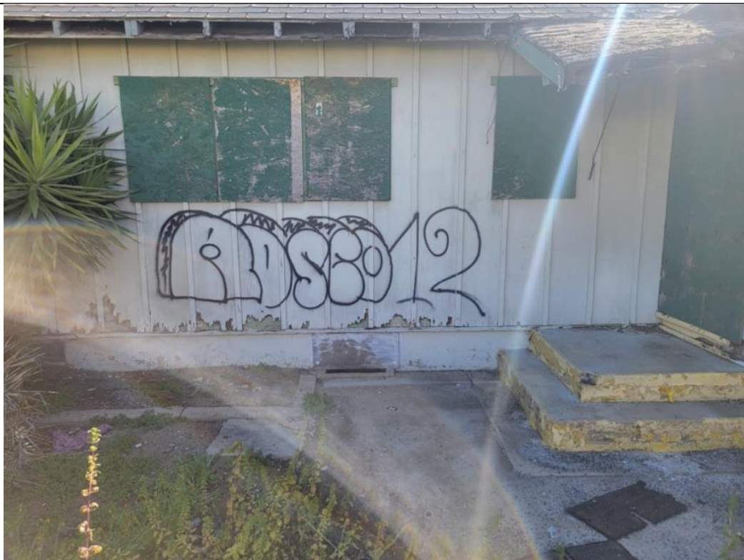
Photograph 4: Barracks, west elevation (rear), graffiti, collapsed porch roof.
