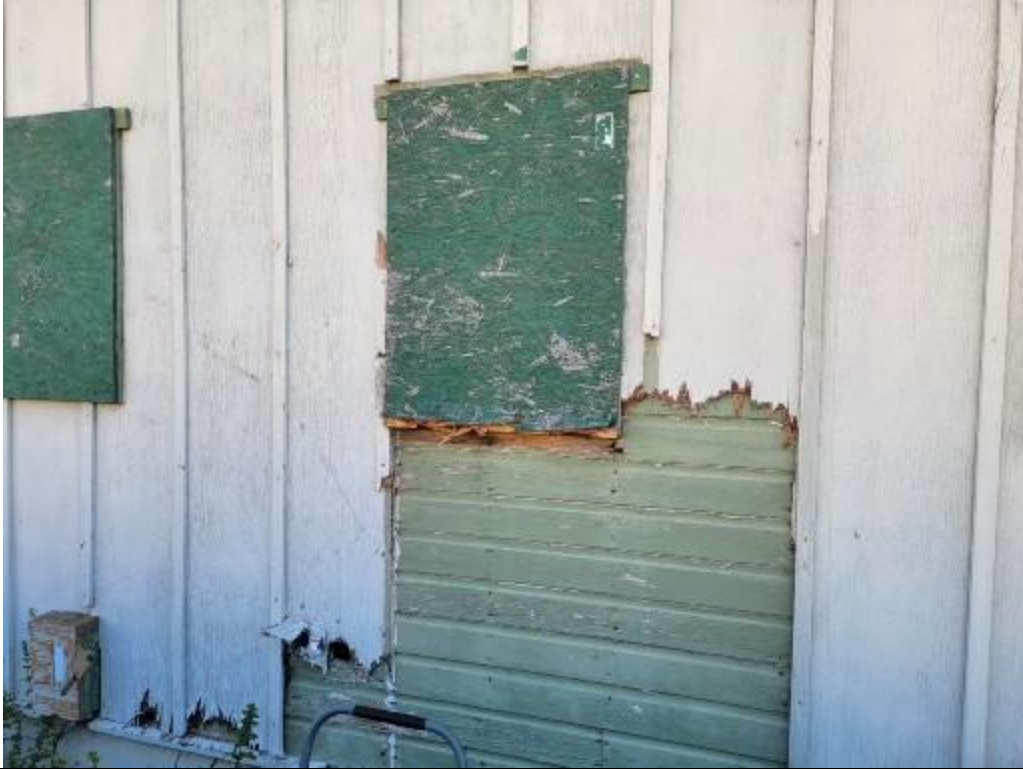
Photograph 5: Barracks, west elevation, missing/damaged exterior cladding.
