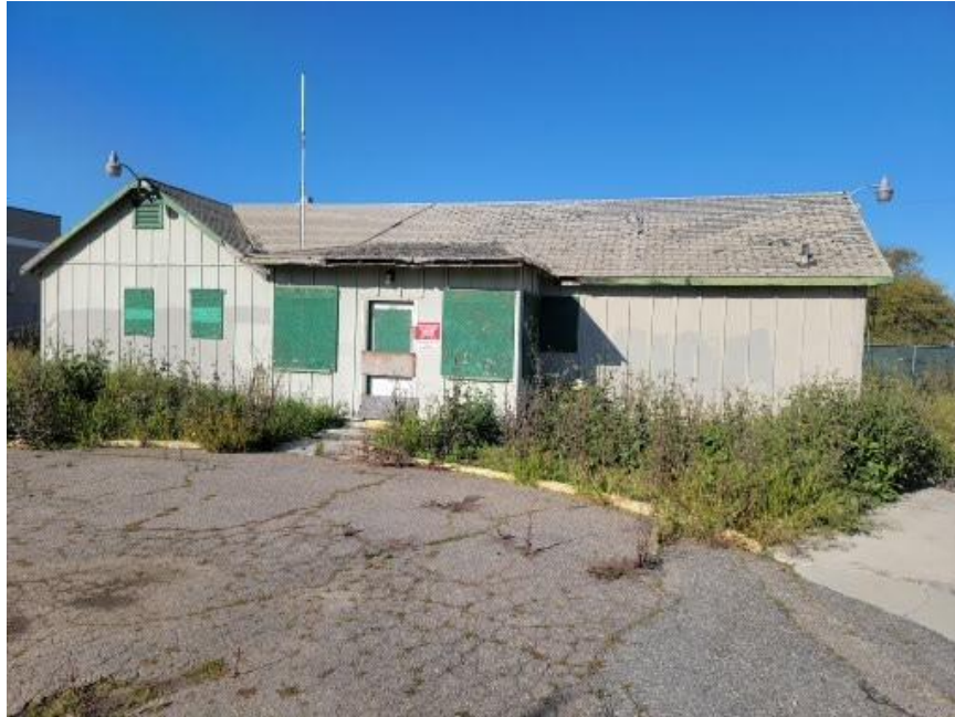
East (front) entrance to Barracks. Boarded windows, fading paint, damaged roof, and modern radio antenna shown.
