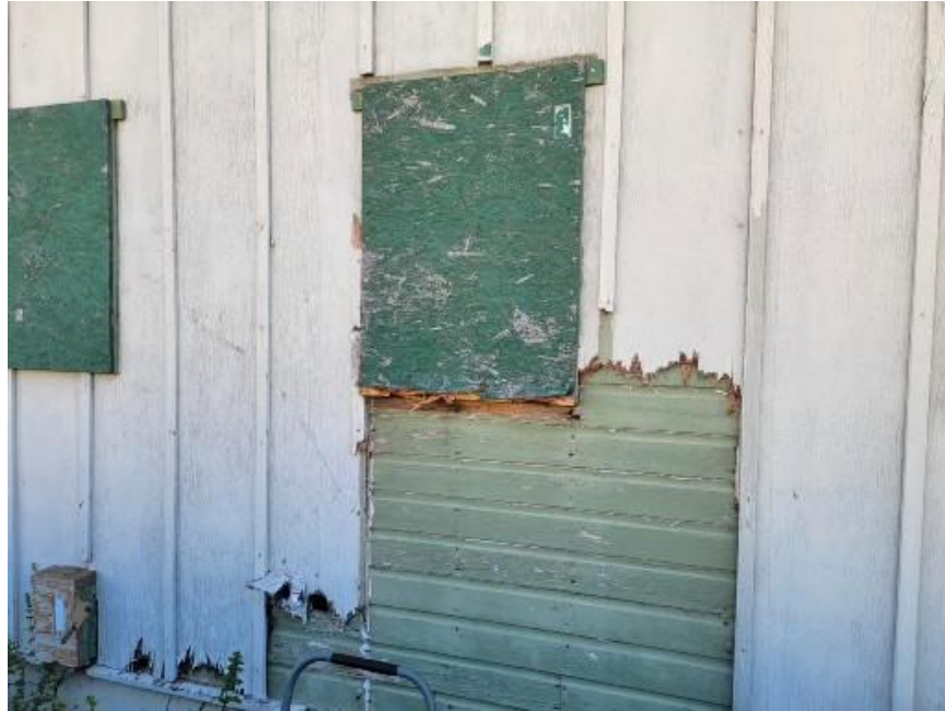
West (rear) face of Barracks with significant missing/damaged exterior cladding.
