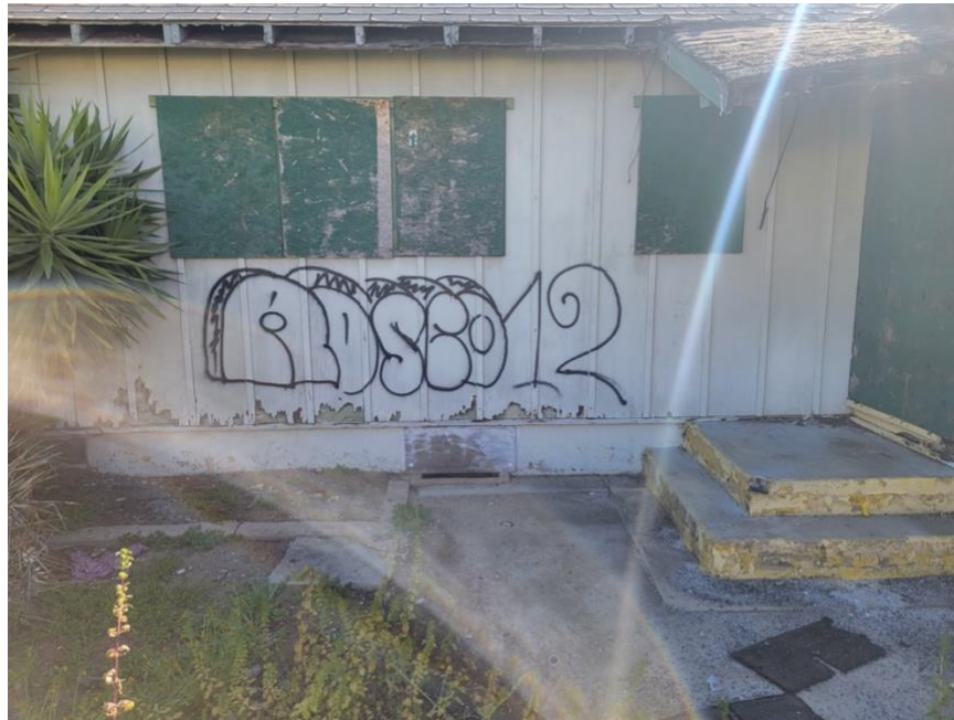
West (rear) face of Barracks showing both modern graffiti and collapsing rear porch roof.
