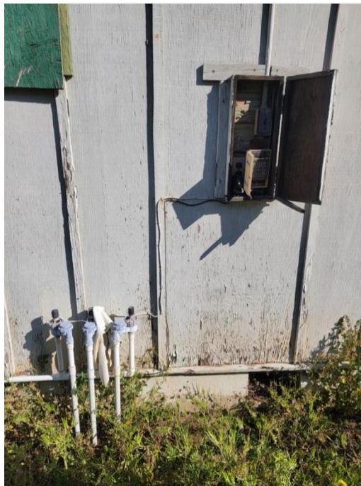
South face of Barracks showing modern surface-mounted sprinkler controller system.
