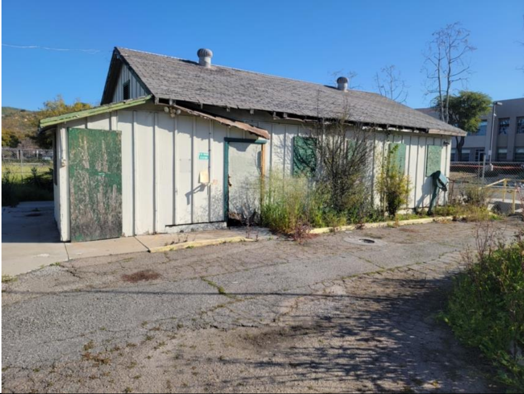
Photograph 7: Garage, south elevation, collapsed and missing fascia.
